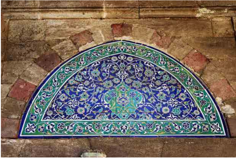
FIGURE 9.18 Cuerda seca tile lunette of the Sultan Selim Mosque in Istanbul (1520s). Photograph by the author.
