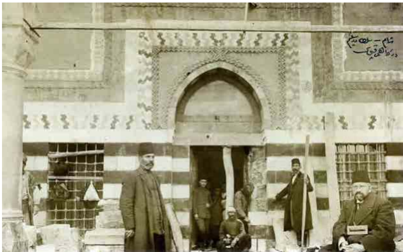
FIGURE 9.7 The Madrasa al-Salimiyya during the renovation: Damascus – The entrance of the dervish lodge of Sultan Selim (Şâm – Sulţân Selîm dergâhı kapısı). Courtesy of Wolf-Dieter Lemke, Berlin.
