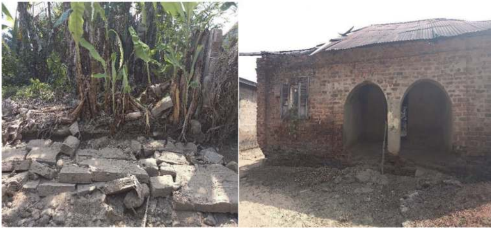
Figure 10. A collapsed fence and an abandoned house with the roof destroyed by the heavy storms.
