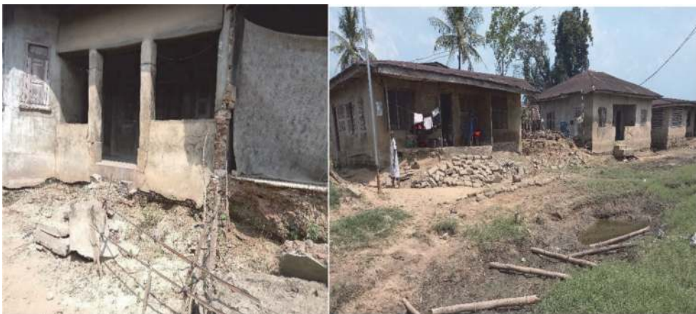
Figure 11. Poorly developed houses, inadequate facilities, and poor living conditions of the residents.
