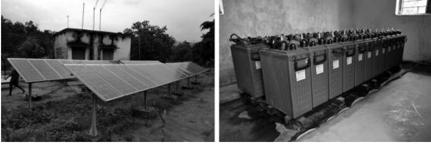
Figure 3.2 Photographs of a mini-grid at the field-site. Notice the solar panels on the ground and a battery-bank inside a control-room.
