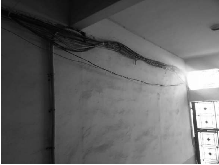
Figure 2.1 Diesel generator wires visible in the foyer of an apartment building in Beirut.
