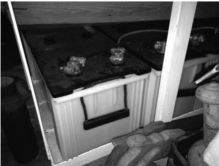
Figure 2.2 Lead-acid batteries mounted on a cradle in the attic of Layla’s house.
