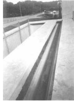
Figure 5.6. Effluent collection launder on the top of an anaerobic filter (Ipatinga WWTP, COPASA, Brazil)
