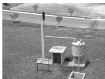
Figure 5.21. View of a hydric seal and gas burner (source: Ipatinga WWTP, Minas Gerais, Brazil)
