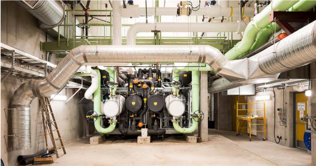
Figure 14.9 A large scale heat pump (~4 MW) extracts heat directly from screened raw wastewater to serve the Southeast False Creek District (courtesy city of Vancouver).
