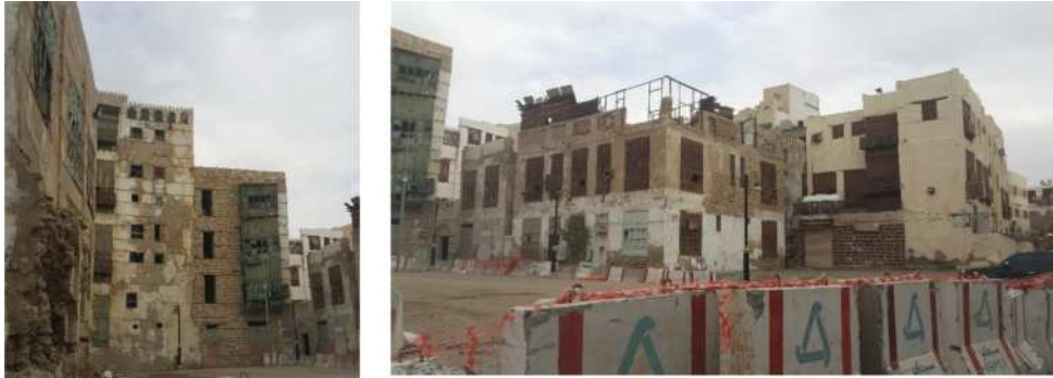
Figure 12. Deteriorated buildings and urban fabric in historic Jeddah.
