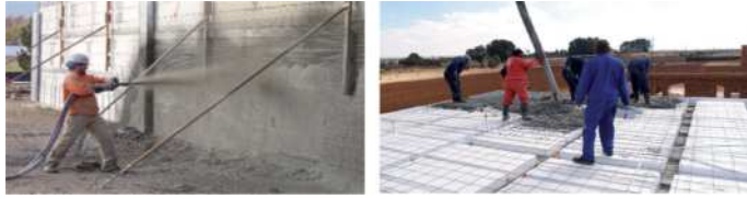
Figure 13. Left, illustrates the shoot Crete and right, illustrates slab construction (designenterprises, 2010), (technopol.co.za, 2017).
