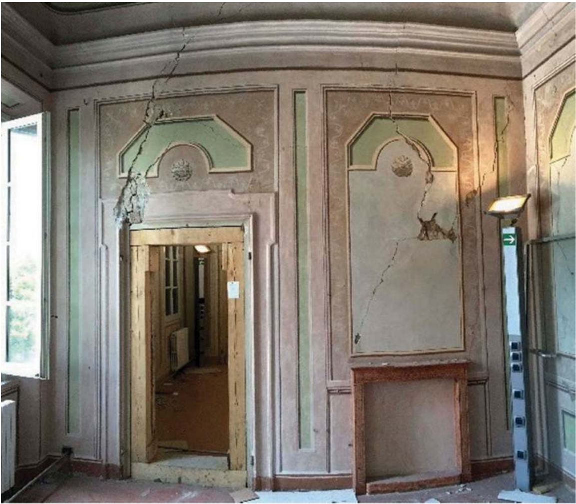
Figure 14. The decorations in the rooms on the main floor of the main body of the building were seriously damaged.
