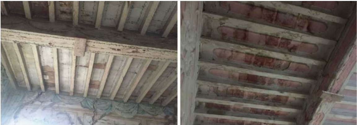
Figure 15. The rooms on the first floor of the western enfilade have wooden ceilings with lime-washed brick tiles and fine decorations that echo the motifs on the walls. There is evidence of water leaking from the roof as a result of the earthquake.
