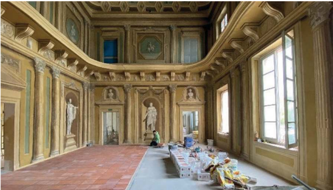
Figure 30. Picture of the Salone during the laying of the terracotta floor after the scaffolding had been removed.
