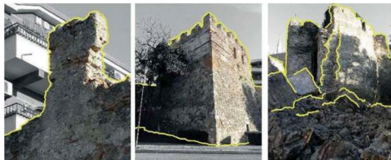
Figure 15. Walls of Durres, serious damage into crenellations.
