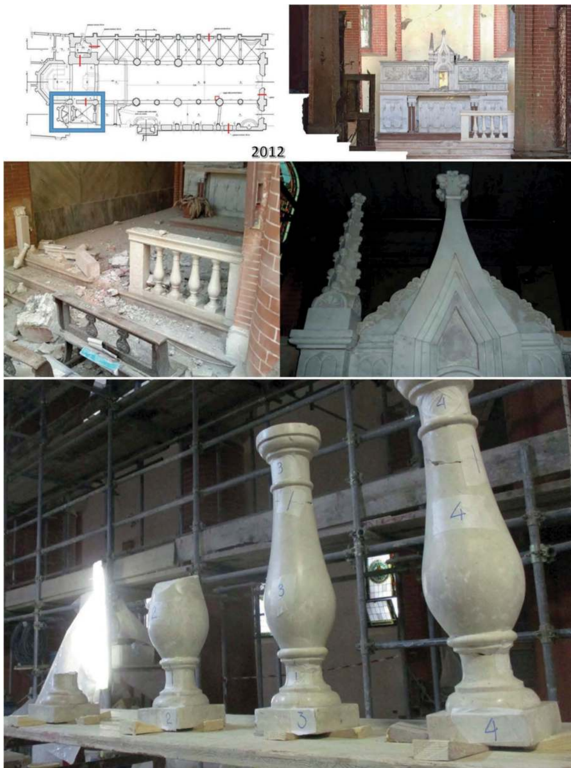
Figure 30. Above, the Altar of the Santissimo, details of the balustrade shattered and the destroyed Tabernacle spire by the collapse. Below, the identification and assembly of the recovered fragments of the balustrade columns.
