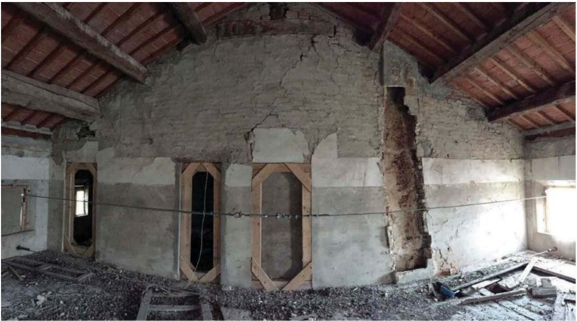
Figure 16. The condition of the rooms in the attic of the western body, which had been uninhabited for decades, was such that even accessing them during the survey was very difficult.
