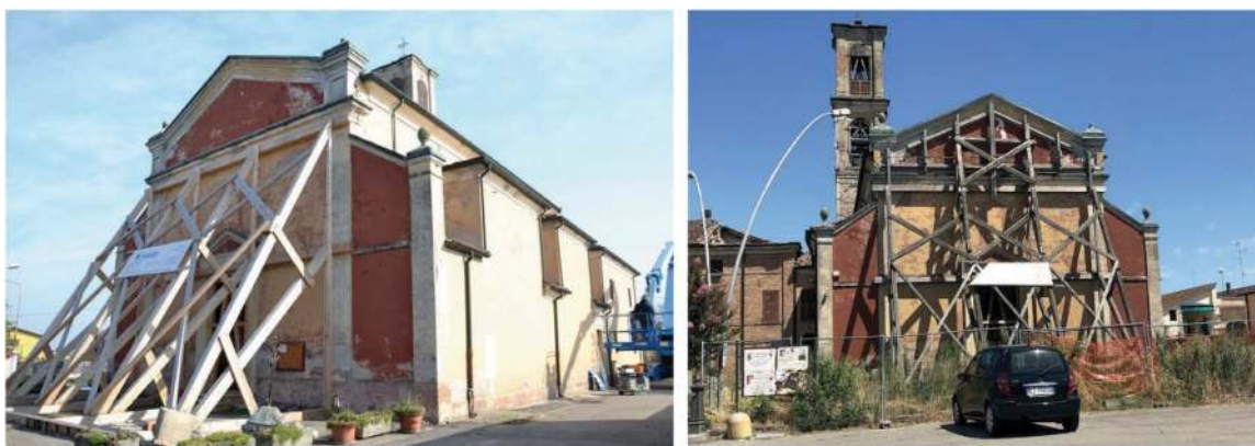
Figure 3. San Michele Arcangelo Church in Bomporto (MO): on the left the wooden rakers installed in 2012, on the right the worsened conditions of the same interventions in 2019.
