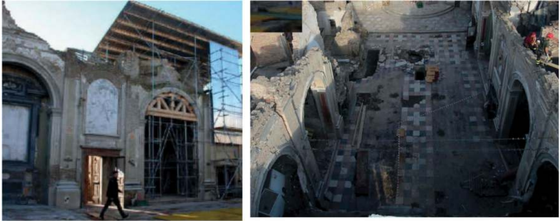
Figure 5. The second phase of the provisional works in the church of San Felice sul Panaro: removal of rubble, shoring of the collapsing walls, partial coverings to protect the decorated areas.
