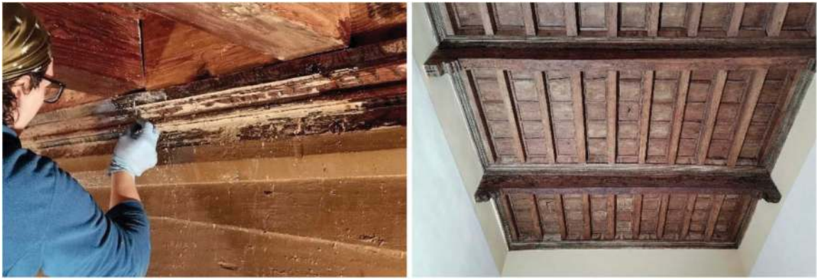
Figure 27. Restoration of the wooden slabs on the ground floor of the 15 th -century part.
