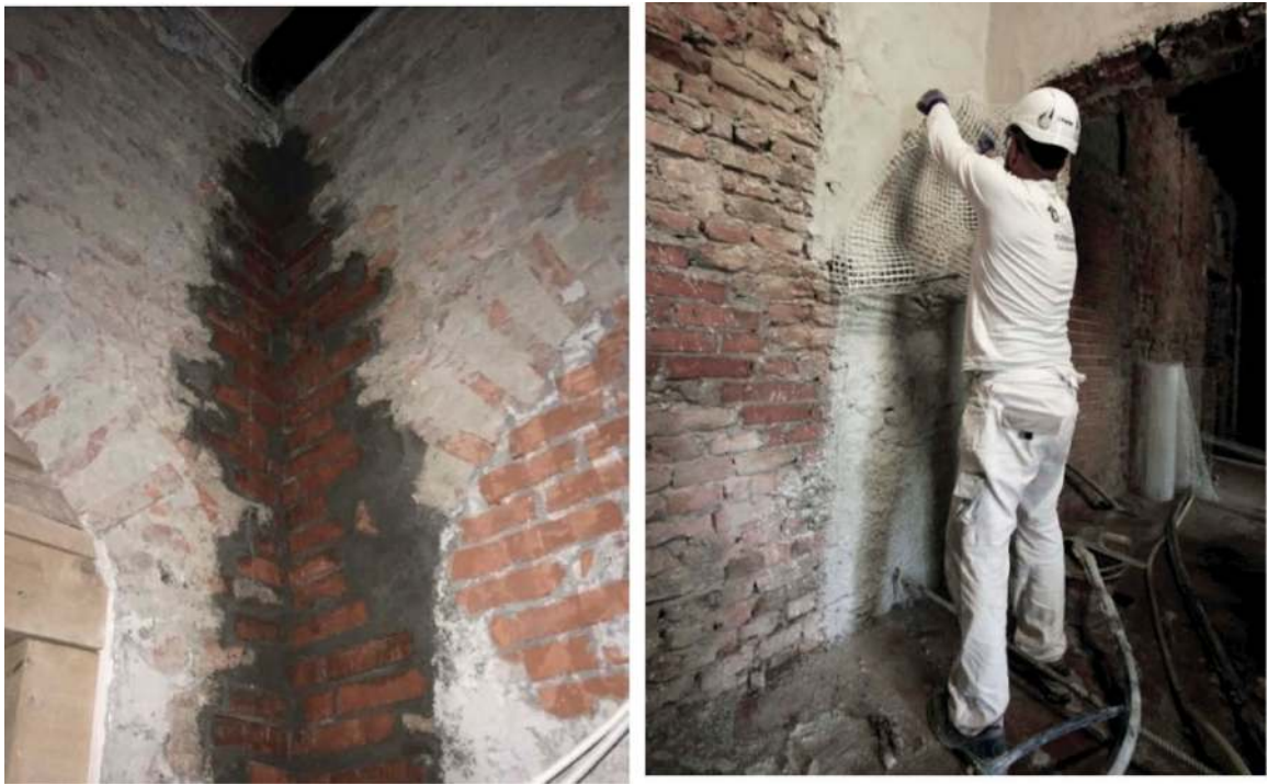
Figure 23. Several masonry walls had little or no tothing between corner walls. Two types of intervention are envisaged, angular like-for-like replacement or the laying of fibreglass fabrics, also placed at an angle, on lime-based adhesion promoters.
