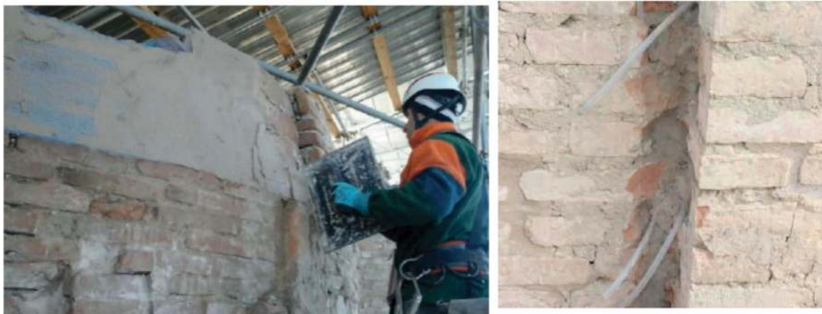
Figure 8. Church of San Felice sul Panaro: thorough operations of masonry walls consolidation.
