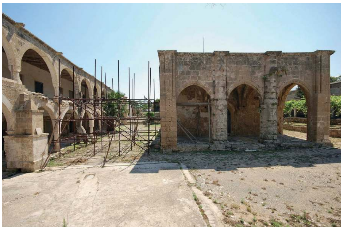
Figure 4. The scaffolding is holding in place the leaning column, urgent intervention is required (photo: A. Camiz, 2014).
