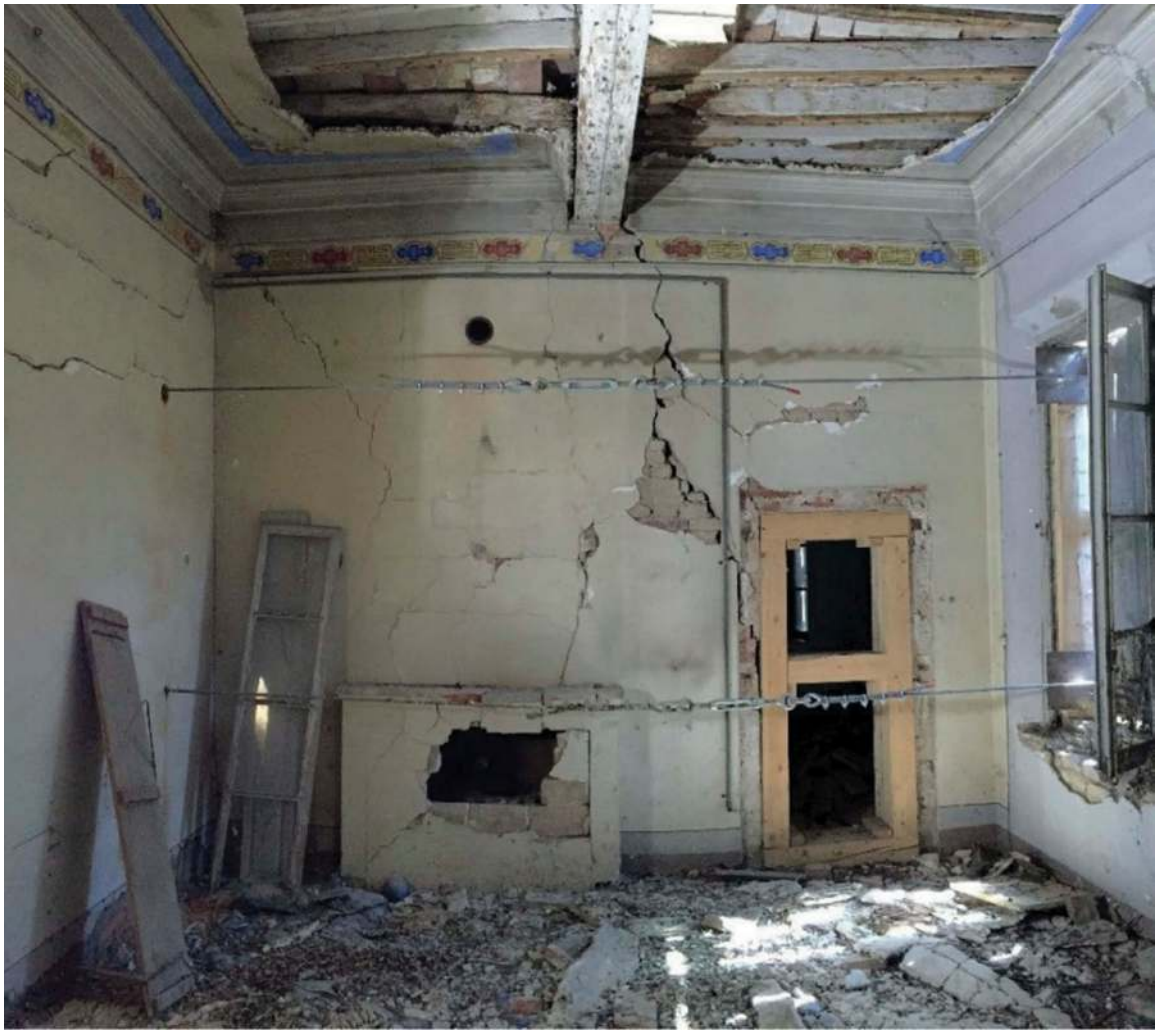
Figure 9. The critical condition in west wing's first floor with deep masonry cracks, partial collapses of suspended ceilings. In the foreground are the chainings for safety measures.
