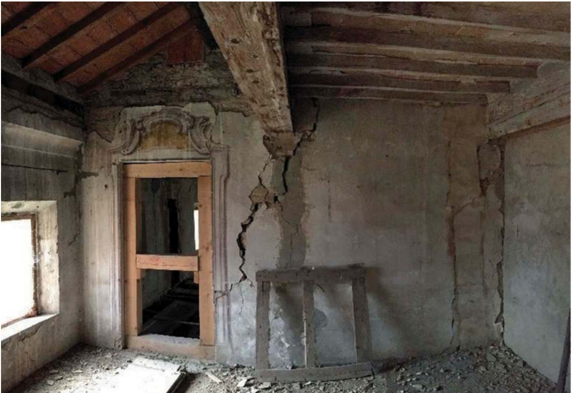
Figure 17. Partial collapses of floors and unsafe portions of the roof represented the main difficulty.
