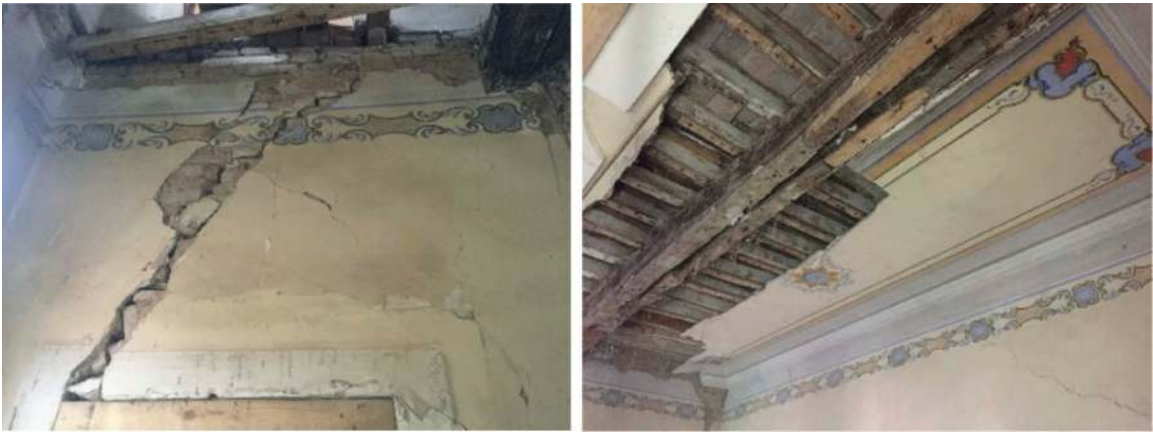
Figure 8. The first floor of the west wing was in a very critical condition, with deep cracks in the masonry, partial collapses of the suspended ceilings and widespread rotting of the wooden beams.
