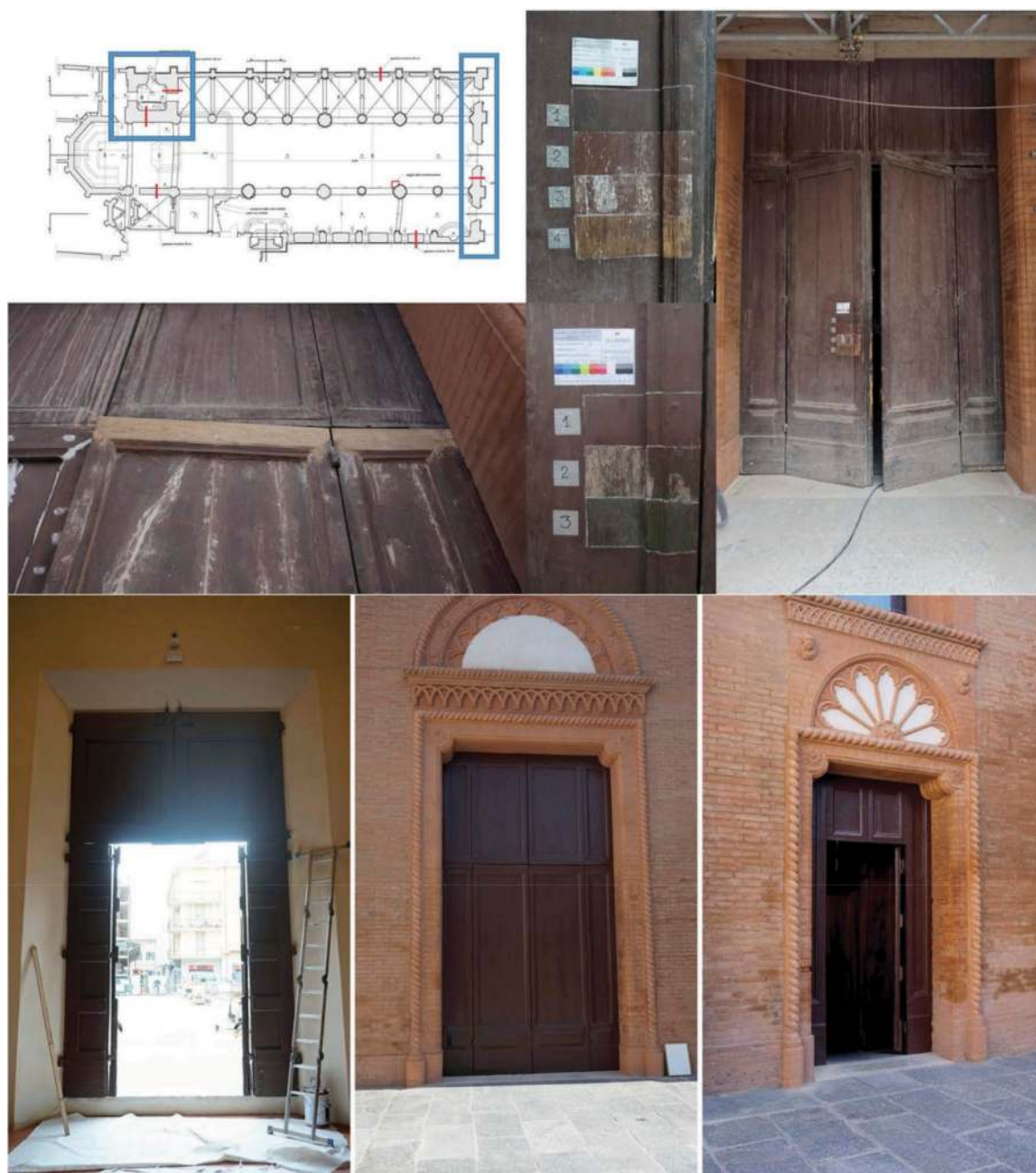
Figure 39. The state of conservation of the main and side entrance doors with images of the stratigraphies conducted to identify the restoration colours and the final state of the doors at the end of the restoration.
