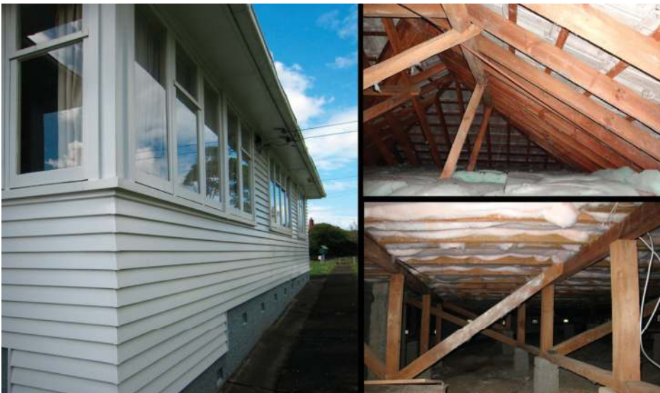
Figure 4. North-west facades , hipped roof cavity (timber rafters with concrete tiles and polyester insulation) and basement cavity (jack studs, sleepers and bracing struts on concrete blocks supporting floor joists with polyester insulation in-between) of the pilot project house in 2012.
