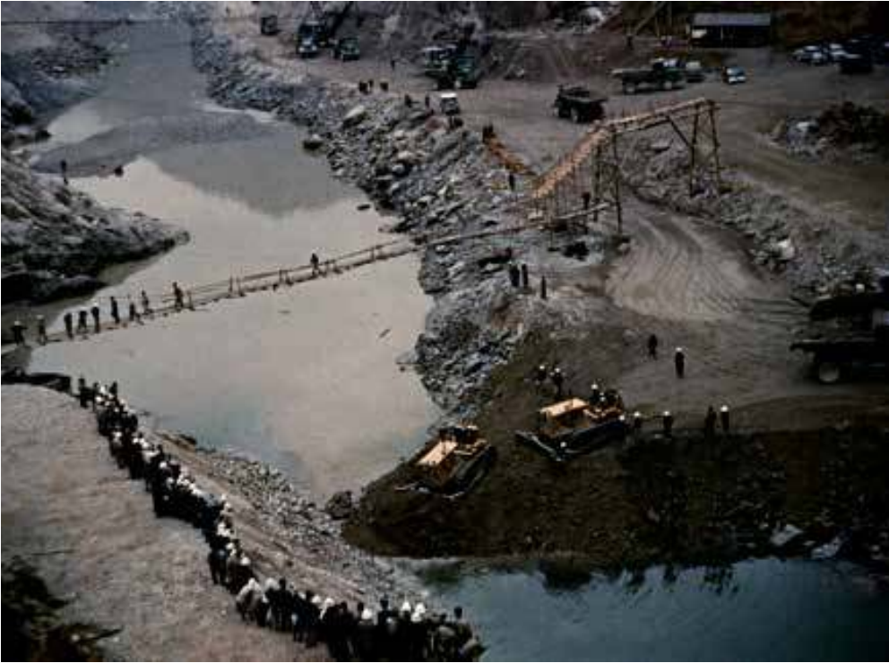
Fig. 8.3. Blocking and diverting the Tenryū River in Sakuma Dam . Picture courtesy Documentary Film Preservation Center, Japan.
