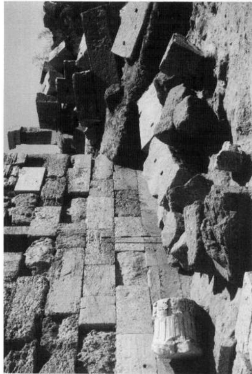
(c) Colonnaded Street: face of north-west outer wall towards the street, showing fine finish of ashlar masonry.
