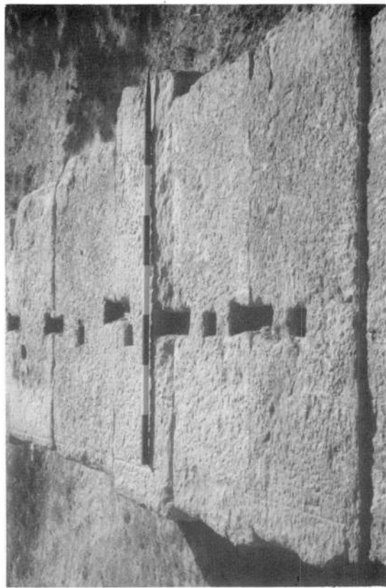
(a) Colonnaded Street: lower foundation course, showing setting-out line and arrangement of cramps.
