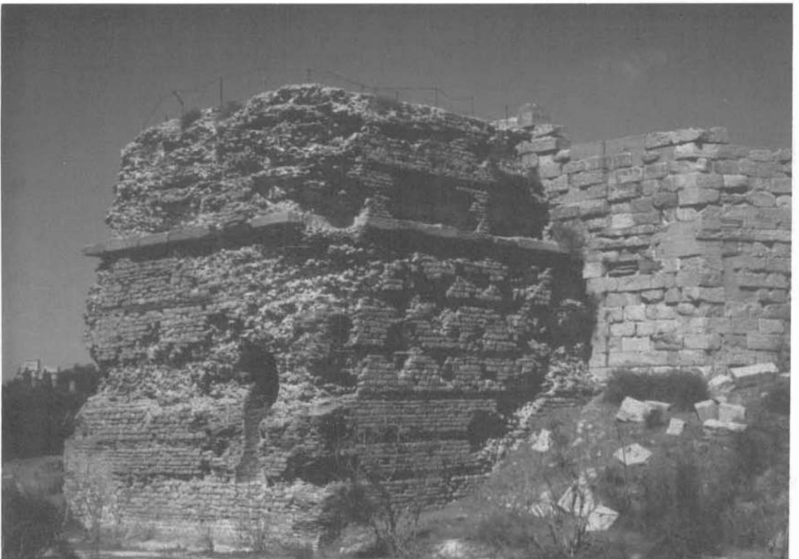
(b) Great Nymphaeum: rear view of the surviving part, showing the concrete of the central hemicycle.
