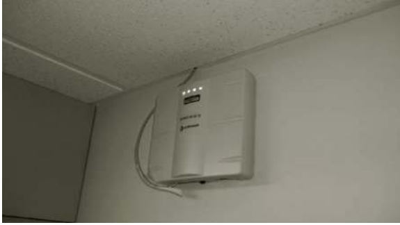
Figure 9.3 Example of poor cable installation.
