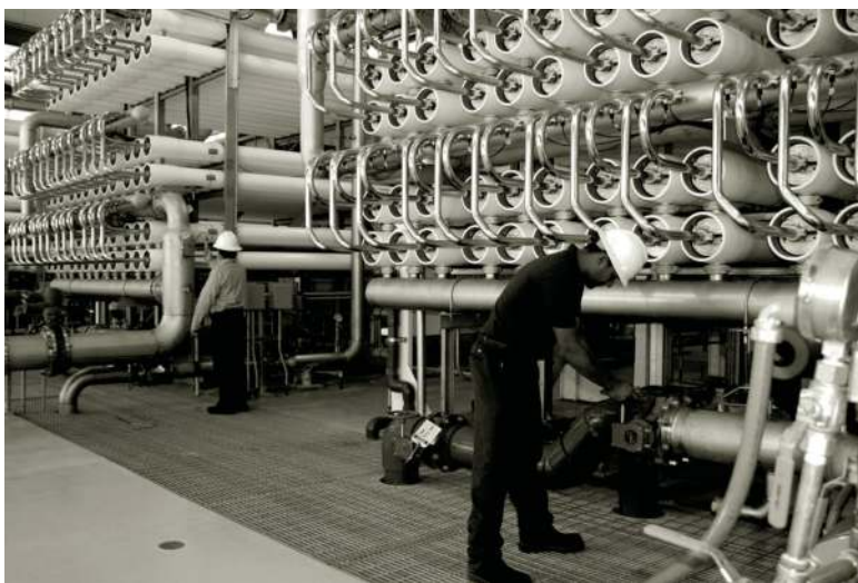
FIGURE 26.8 El Paso water utilities desalination plant. (Courtesy of El Paso Water Utilities.)
