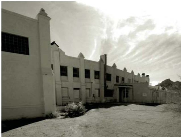
FIGURE 16.6 The boarded Ajo hospital, one of many large public buildings funded by the mine; others are only partly occupied.
