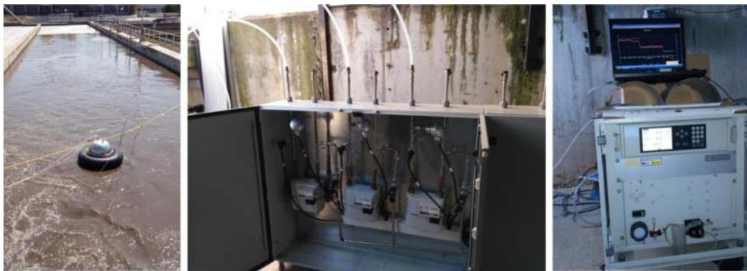
Figure 5.7 Floating hood (configurations C and E in Figure 5.6) and associated equipment for measuring off-gas flowrates and off-gas concentrations. Photos courtesy of Dr. Maite Pijuan (ICRA Catalan Institute for Water Research). These figures were published in Journal of Cleaner Production , Vol number 212, A. Ribera-Guardia, L. Bosch, L. Corominas, M. Pijuan, Nitrous oxide and methane emissions from a plug-flow full-scale bioreactor and assessment of its carbon footprint, Page Nos 162–172, Copyright Elsevier (2019) and in Science of the Total Environment , Vol number 493, A. Rodriguez-Caballero, I. Aymericha, M. Poch, M. Pijuan, Evaluation of process conditions triggering emissions of green-house gases from a biological wastewater treatment system, Page Nos 348–391, Copyright Elsevier (2014).
