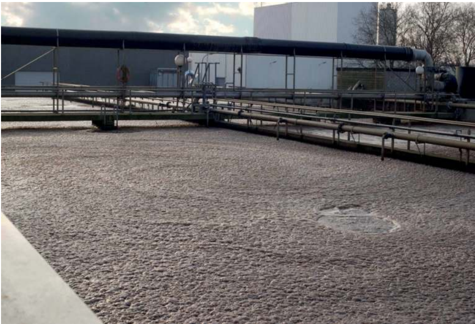
Figure 9.8 Activated sudge tank of WWTP Ecco Dongen (Photo: Moussa M.S.).
