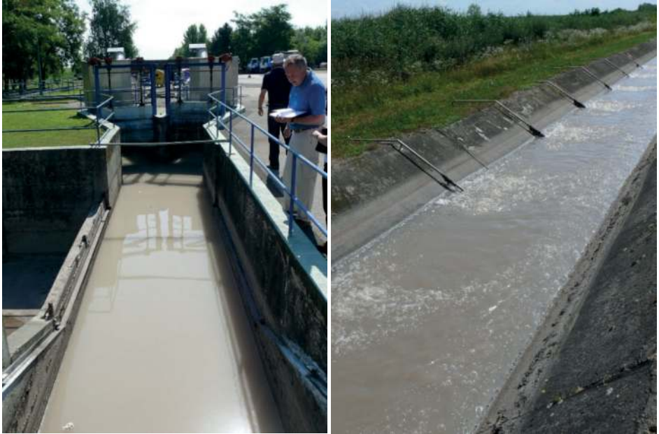
Figure 13.2 Channel connecting the primary and secondary treatment at WWTP Varaždin (photos: Meijer S.C.F.).
