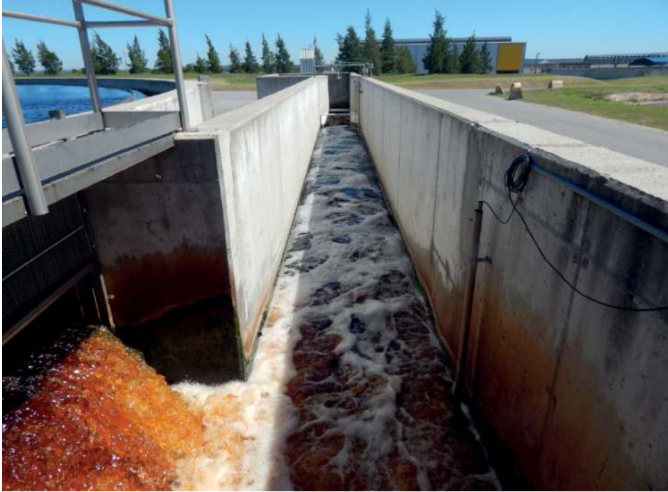
Figure 16.6 Secondary treatment at the pulp mill WWTP of study: Effluent to Uruguay River (Photo Bentancur S.).
