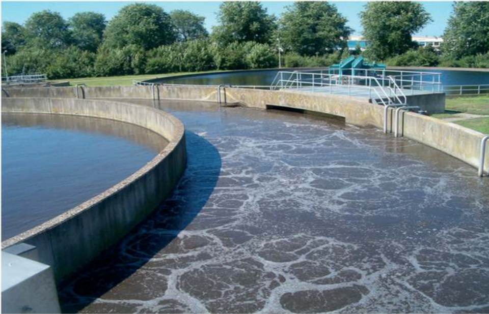
Figure 3.12 Activated sludge tank at WWTP Haarlem Waarderpolder with anoxic inner ring and outer aerobic ring and overflow to secondary clarifier (Photo: Brdjanovic D.).
