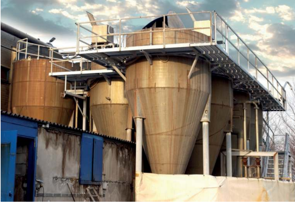
Figure 9.7 Primary settling tanks of WWTP Ecco Dongen (Photo: Moussa M.S.).
