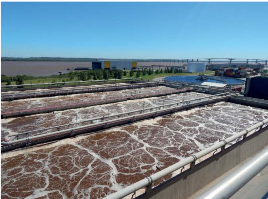
Figure 16.5 Secondary treatment at the evaluated pulp mill WWTP: Conventional aerobic activated sludge system (Photo Bentancur S.).
