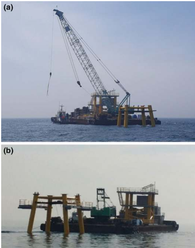
Fig. 2.14 (a–b): Deployment of the first wind farm foundation at the co-location wind farm project in the south-west of South Korea. a Foundation during mooring procedure; b preparation of the foundation for potential multi-uses. Modified after KEPCO and KIOST (2016)
