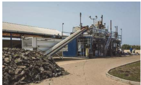
Figure 2.11 The omniprocessor faecal sludge treatment system in operation in Dakar, Senegal (photos: UKZN PRG and Sedron Technologies).
