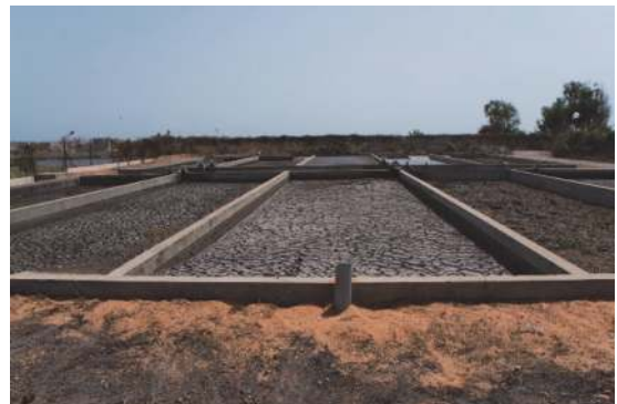
Figure 4.3 Drying beds at Niayes FSTP, Dakar, Senegal (photo: Eawag).
