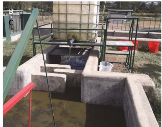
Figure 4.12 A) a Sanivation employee washes detergent, salt, and particulate residue from a geotextile using a high-pressure water rinse and B) example of a conditioner dosing configuration: one dosing port followed by mixing with baffles (photos: Sanivation).
