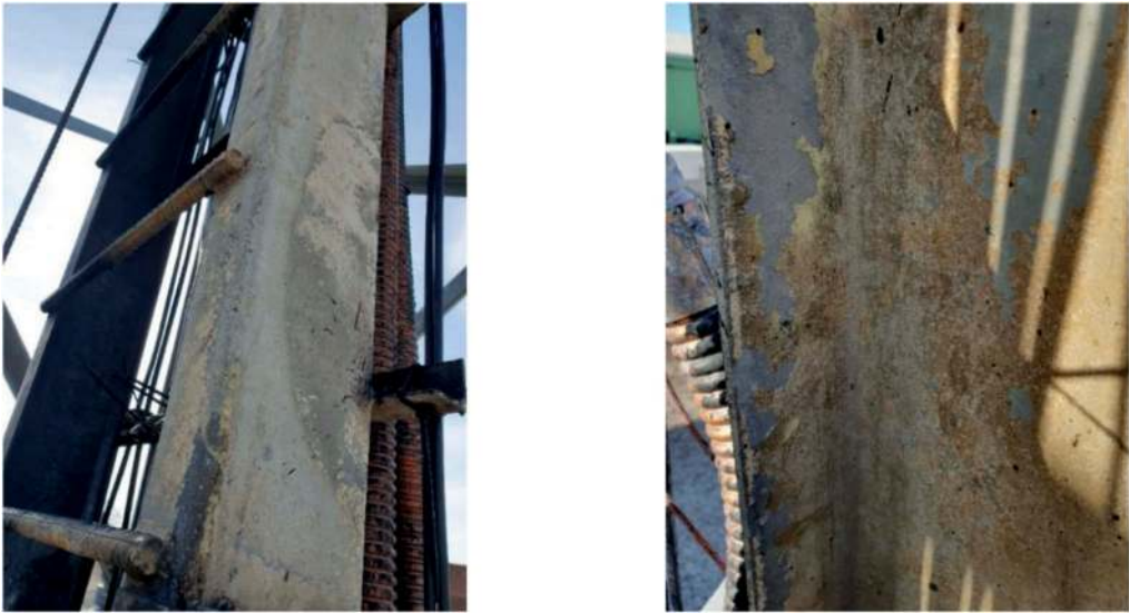
Figure 6. The effect of elevated temperature on components of the ladder rails (D-8 element).
