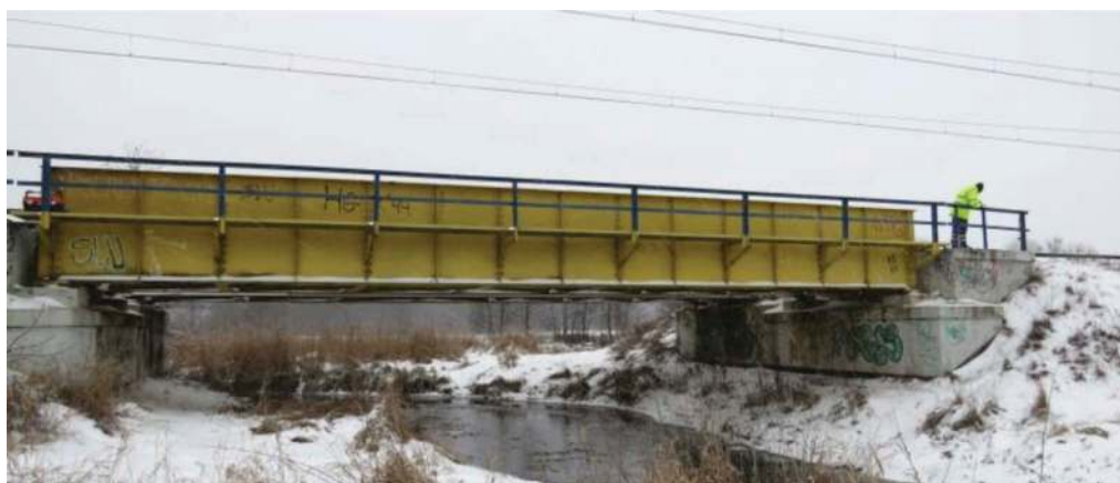
Figure 1. View of the span of the railroad bridge on km 207.887 of the railway line No. 7 Warszawa Wschodnia – Dorohusk.
