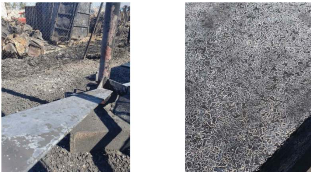
Figure 7. The blue temper on bracing sections in the bottom segment of the tower.
