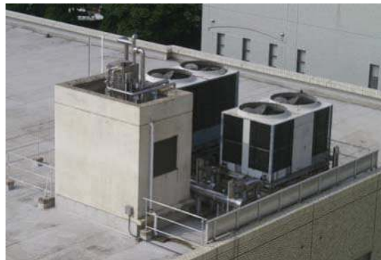
Fig. 14. Heat pump - chiller units
