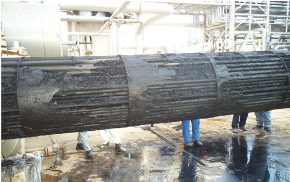
Figure 1. Fouling of heat exchangers.
