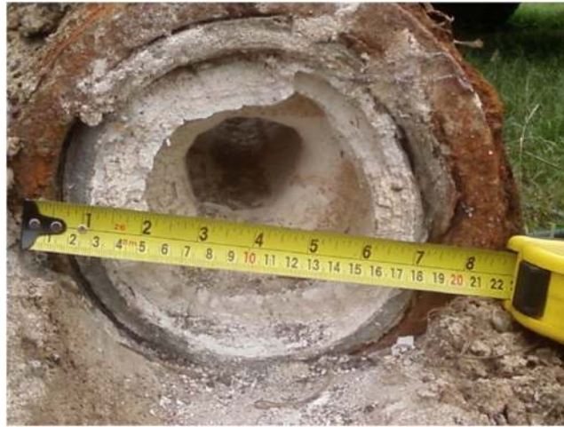
Figure 10.3 Unwanted inorganic scale within water pipework.
