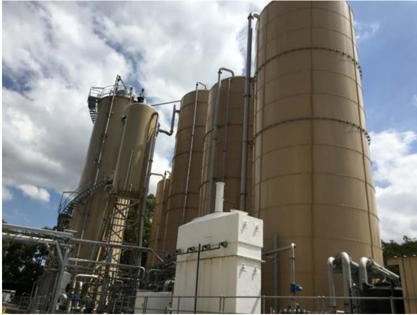
Figure 5.17 Example of an internal circulation (IC) reactor and associated infrastructure installed at a brewery.
