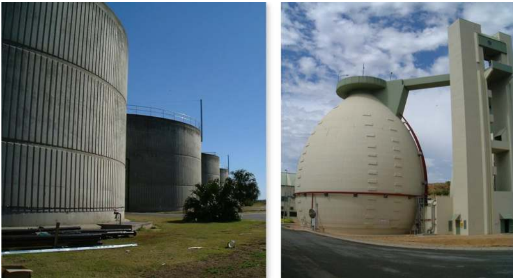
Figure 5.8 Examples of mixed liquor anaerobic digesters installed at municipal wastewater treatment plants in Australia.
