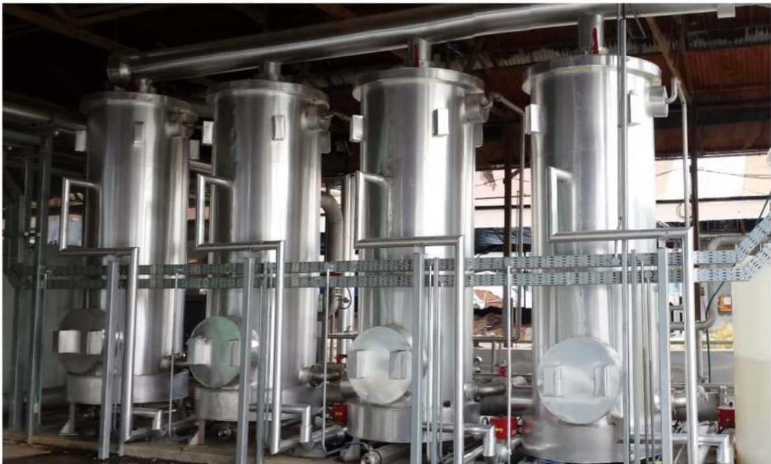
Figure 10.24 Operating ammonia recovery facility treating the digestate from a large poultry manure anaerobic digester (courtesy of Anaergia).
