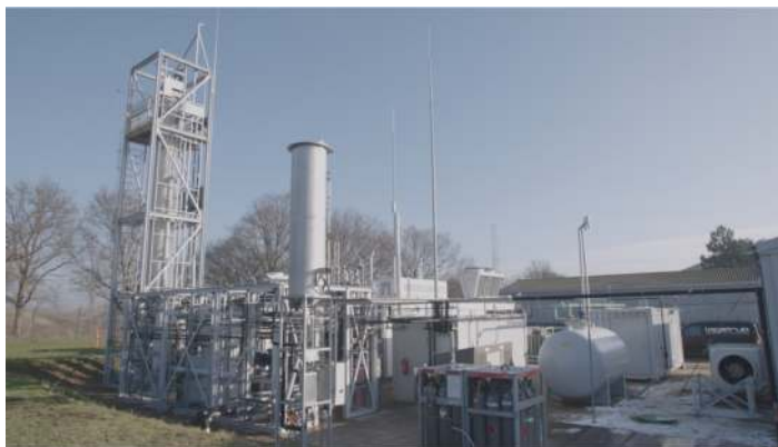
Figure 6.6 Picture of a 1-MW power-to-methane system at a wastewater treatment plant. The stirred bioreactor with bubble formation in a column is on the left. This picture was taken at Electrochaea's patented BioCat plant in Avedøre, Denmark, which is a demonstration-scale system to store biogas as renewable natural gas in the Danish natural gas grid.
