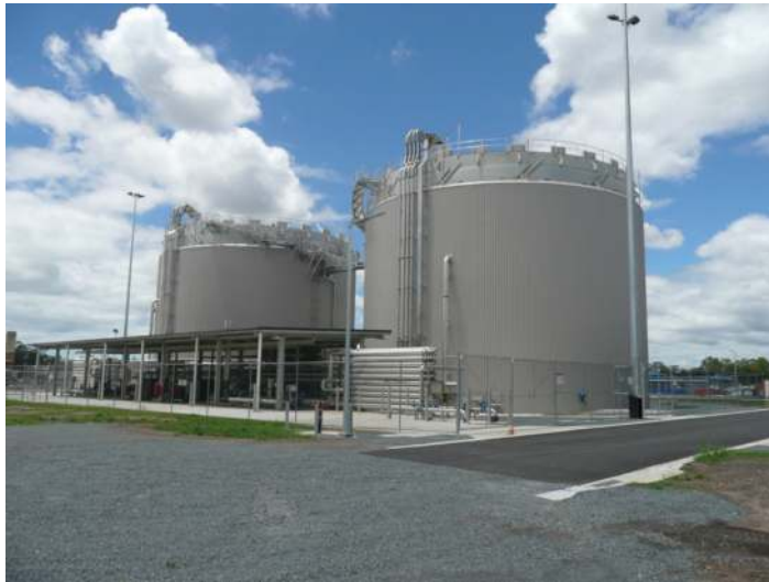
Figure 5.18 Example of two continuous mixed liquor digesters installed at a sewage treatment plant to stabilize waste activated sludge (Gloag et al. , 2014).
