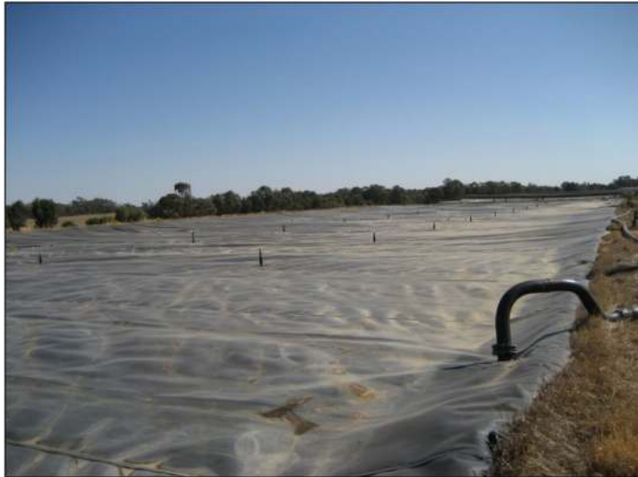
Figure 5.16 Example of a covered anaerobic lagoon installed at a rural pig production facility (Gopalan, 2013).
