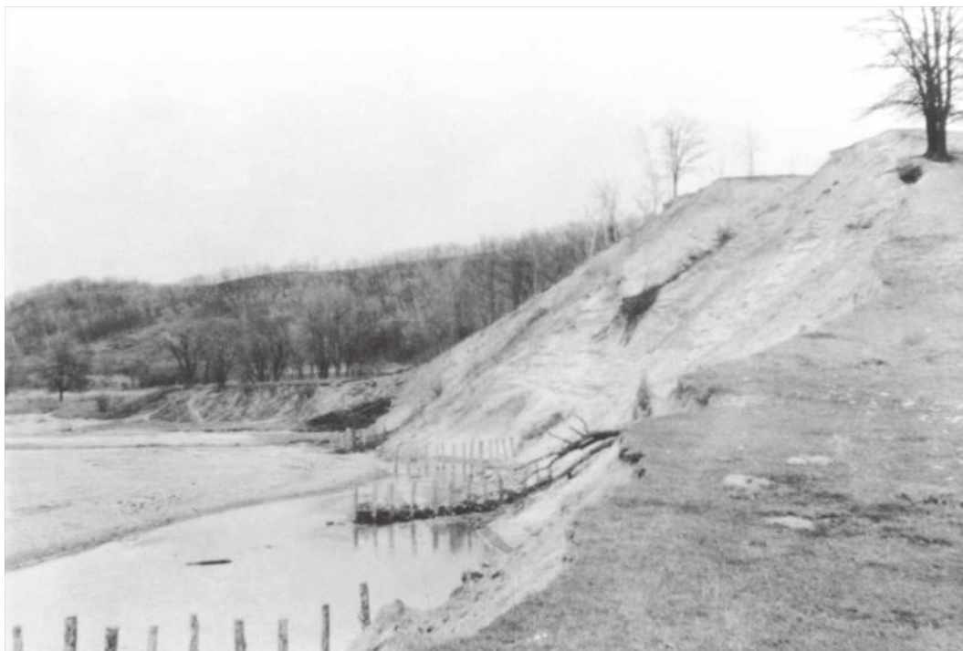
Figure 2.16 CCC project to stabilize high Pleistocene terrace undercut by stream. Exact location unknown but probably Trempealeau Co., WI, late 1930s. SCS Photo.
