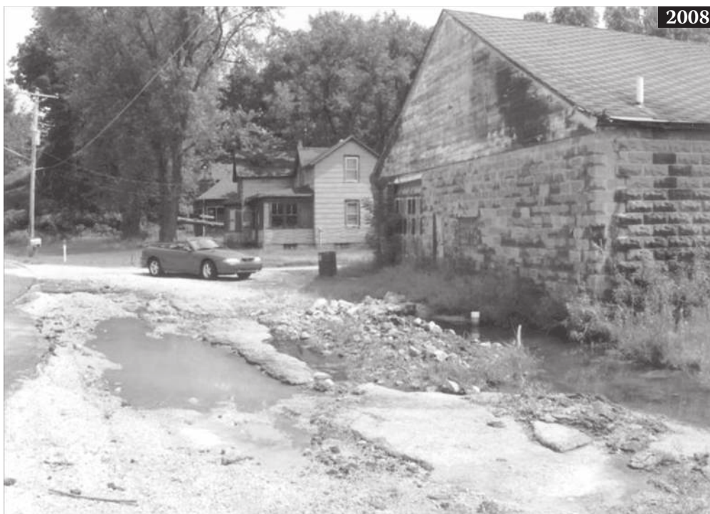
Figure 7.8 (Continued) July 2008. Two large floods had passed though in the preceding 10 months and the building was abandoned and derelict.
