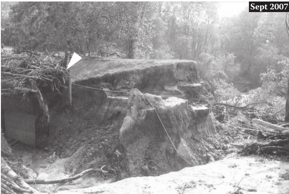
Figure 8.8 Proksch Coulee Trench, looking downstream at the dam and drop structure built in 1936 by Soil Conservation Service to stabilize gully, 2 mi (3 km) east of Stoddard WI ( P > 12 in., or 30 cm). Viewer stands on reservoir fill. Top: Dam and drop inlet, looking downstream, July 2007. Arrows point to top-right corner of drop structure. Note sediment filled to level of drop inlet (see Figure 4.10). Bottom: Breached dam, September 2007. Note drop inlet to left covered and blocked with woody debris. Gully in foreground extends about 200 ft (60 m) upstream in accumulated sediment. Bottom of gully visible in right background is about 30 ft (9 m) lower than dam. (Photos credit: Edyta Zygumunt.)
