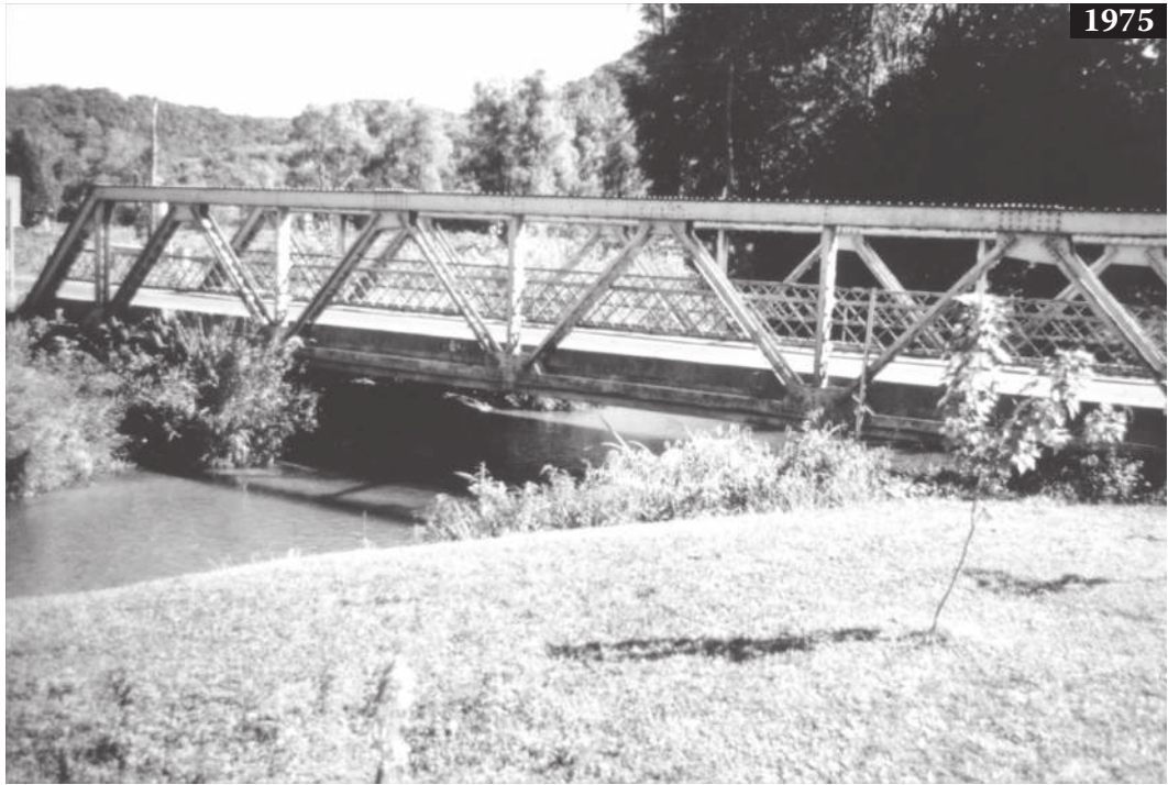
Figure 7.4 Continued 1975: Replacement bridge at the same site as above, looking southeast (upstream). The newer bridge sat about 1 ft (30 cm) higher than the old bridge but had only about 4 ft (1.2 m) of clearance above the water in 1977. The 2011 water level here is 10–12 ft (3–4 m) higher than in 1914.
