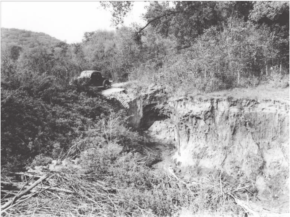
Figure 4.2 Gully heads (overfalls) threatening economic activity in the late 1930s. Top: A threatened farm possibly in Trempealeau Co., WI. Bottom: A threatened roadway in Wabasha Co, MN, 2 mi (3 km) SW of Weaver.
