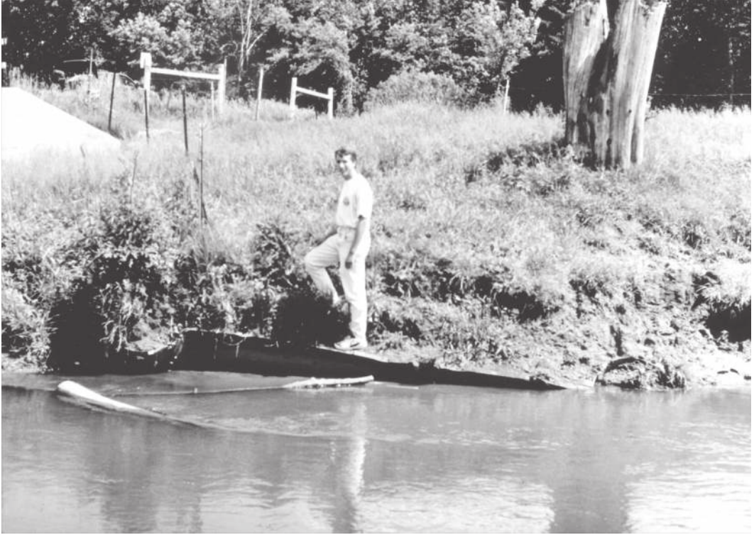
Figure 7.23 The south abutment of an old Dodson Hollow Road bridge over Coon Creek (SE1/4, Sec 22, T14N, R6W, Vernon, Co., WI). This bridge was replaced in 1926 as the creek rapidly aggraded, and the abutment was later buried in the floodplain. When built, probably in the early 1900s, this abutment was at least 10 ft (3 m) above the water. A small lateral shift by the stream in 1993 exposed the old abutment. The newest bridge (c. 1990) is seen to the far left.
