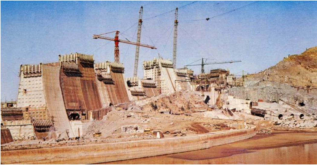
Fig. 130 Photographer unidentified/Department of Information [?]: 'General view of the Hendrik Verwoerd Dam under construction.', Taming a River Giant. The Story of South Africa's Orange River Project , c. 1967–1970.
