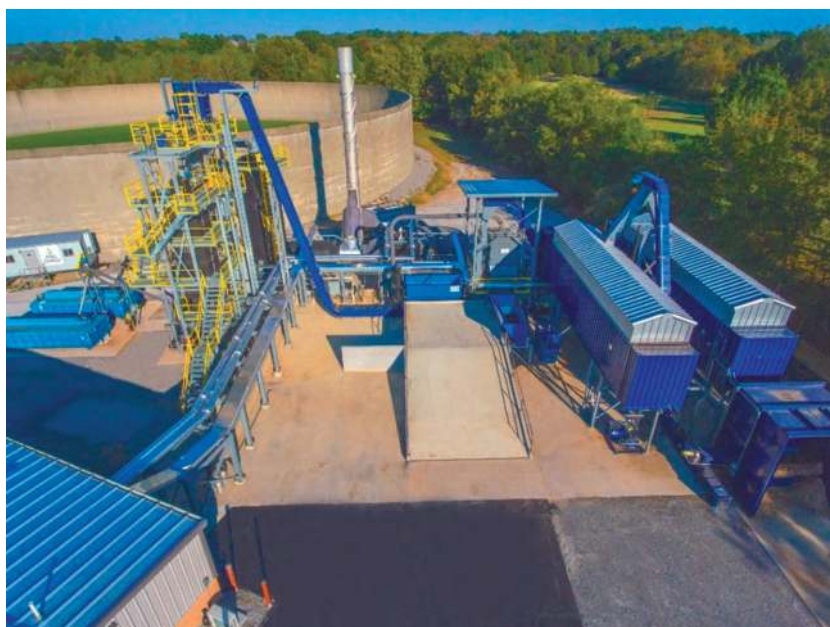
Figure 16. Coca-Cola recycling plant at Kyambogo-Kampala Uganda [55].
