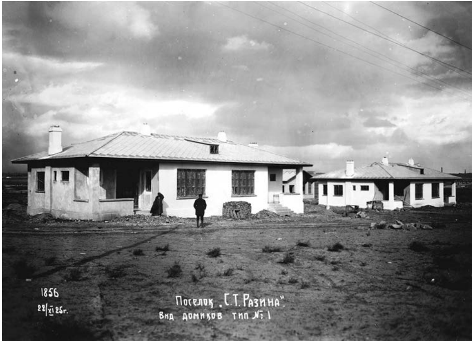
Figure 2.10. Type I houses under construction, Azneft Stepan Razin settlement, Baku, Azerbaijan, November 22, 1925. Architects: Aleksandr Ivanitskii, Viktor Vesnin, Leonid Vesnin, et al. Canadian Centre for Architecture, PH1998:0011:014. Gift of Howard Schickler and David Lafaille.
