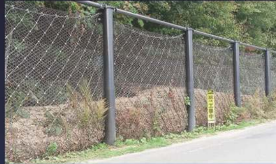
SLOPE GUARD FENCE: Slope failure protection fence caught soil of slope failure caused by a heavy rain.
