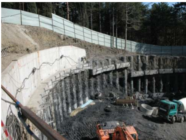
Fig. 4 Stages of construction: pit when arranging the 2nd tier of beams for anchor fixing
