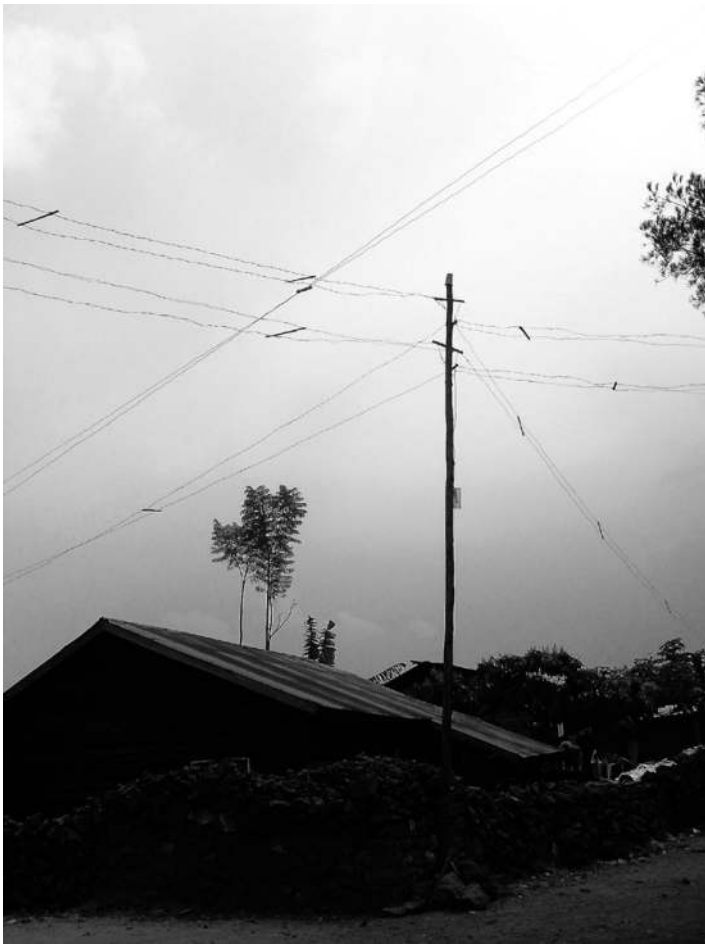
Figure 6.3 Street in Goma, self-made electrical line, photographed 27 July 2010
