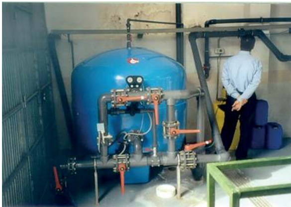
Figure 17 Sand filter. Gran Canaria, Spain.
