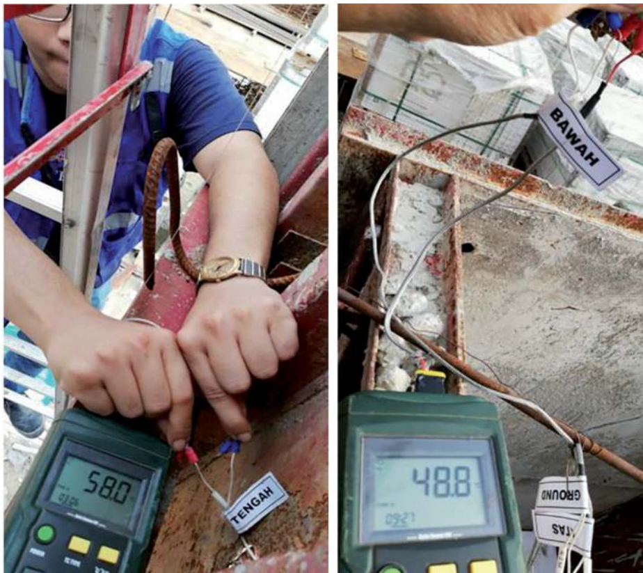
Figure 18. Bioconc LHC mock up thermocouple monitoring.
