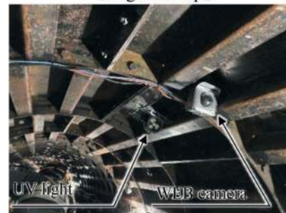
Photo 5. Status of equipment set up at site2.
