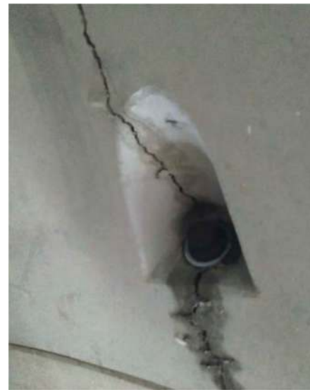
Figure 7. Cracking after the bolt tightening into its pocket.
