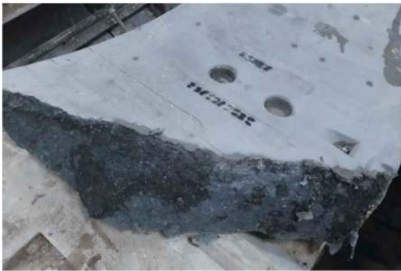
Figure 2. Detail of a SFRC segment that broke in half during installation.
