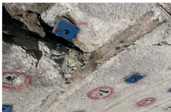
Figure 2. Deformation situation of the support which occurred.
