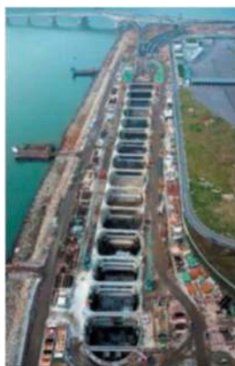
Figure 6. Caterpillar-shaped cofferdam for southern cut and cover tunnel (Schwob, a, et. al, 2020).
