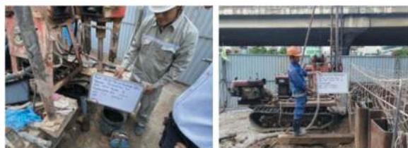
Figure 10. Field permeability test on Chemical grouting and Core sampling on Jet grouting.
