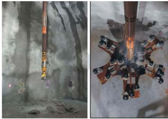
Figure 15. Pilot holes and raise borer machine for the excavation of the Avrieux shaft.
