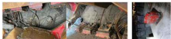
Figures 11, 12 & 13. Anchors in the cutterhead chamber (left and center) & Tungsten knives on the cutterhead (right).
