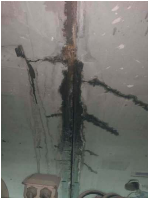
Figure 9. Cracks in the area of the bolt insert (on the upper left) and in the circumferential joint in both segments.
