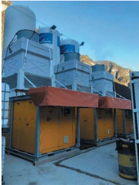
Figure 10. Brine storage plant.
