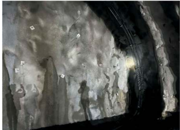
Figure 3. RRS installed close to the face of a tunnel where the tunnel face is also supported by bolts & shotcrete.
