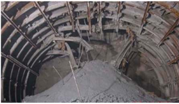
Figure 5. Failure of high-capacity tunnel support.
