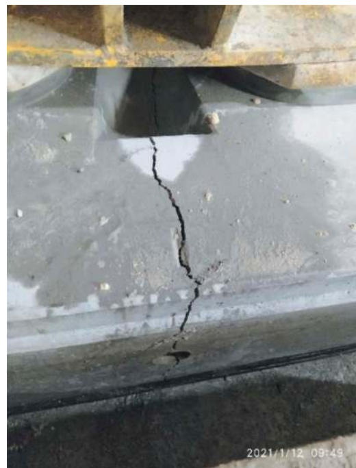
Figure 11. Crack that occurred when the segment was to be installed.
