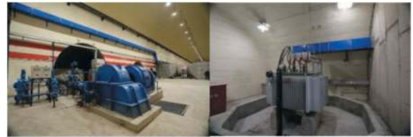
Figure 5. Power generator in the underground fan room.
