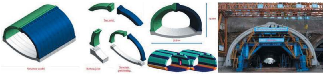
(a) Schematic diagram and on-site construction photo of the prefabricated highway tunnel structure on Xinsen Avenue in Jinfeng Park, Chongqing
