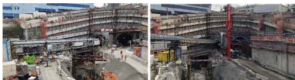
Figures 15 & 16. TBM Launching area at Maungawhau, a busy area with several interfaces.
