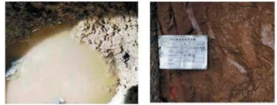
Figure 8. Inverted arch water accumulation and tunnel face seepage water.
