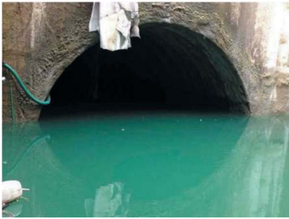
Figure 4. Flooding of the executed works.
