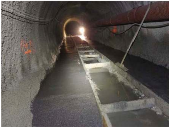
Figure 2. Water in main collector.
