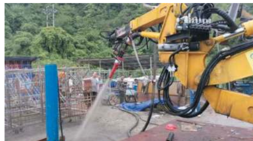
Figure 15. Concrete shotcreting operation of the complete equipment for treating the defects of operating tunnels.
