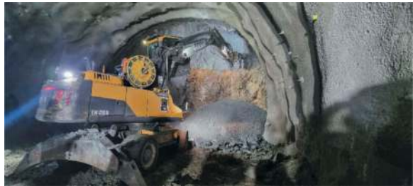
Figure 6. Excavation with drum head. The left part of the tunnel face is supported by sprayed concrete, and the right part shows the weathered rock (brown material) and clay moraine (grey material on top).
