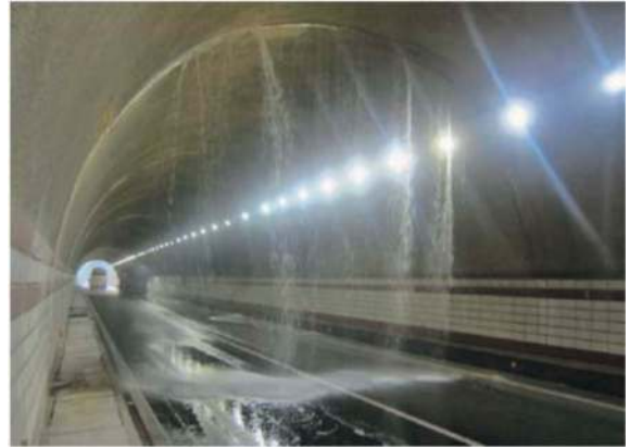
Figure 15. Water curtain disease formed at construction joints.
