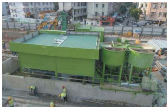
Figure 2. Mechanical dewatering and drying equipment constructed on site by Shenzhen Metro.
