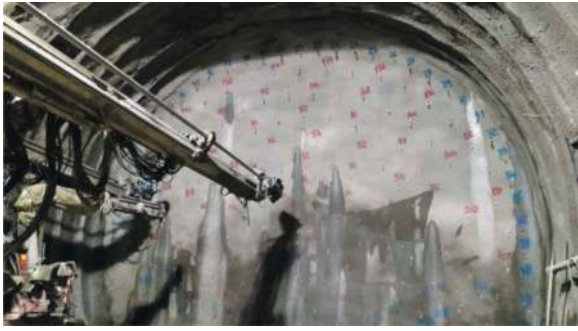
Figure 12. Section C1: Blue marks truncated cone 'umbrellas', red marks core face reinforcements.
