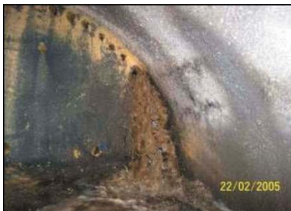
Figure 6. High water ingress during excavation.
