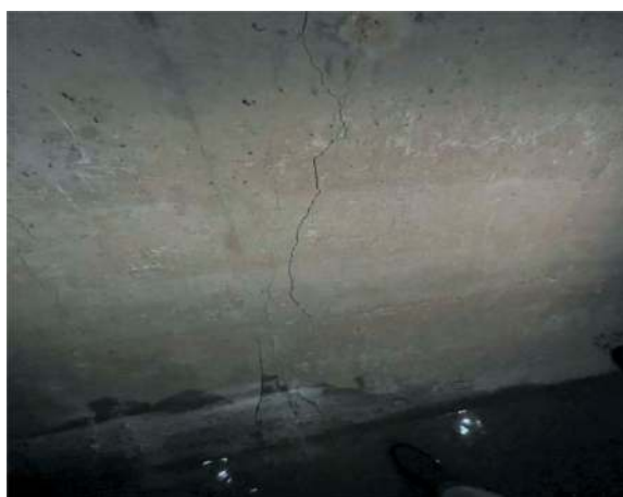
Figure 13. Cracks in the lining of the conduit.
