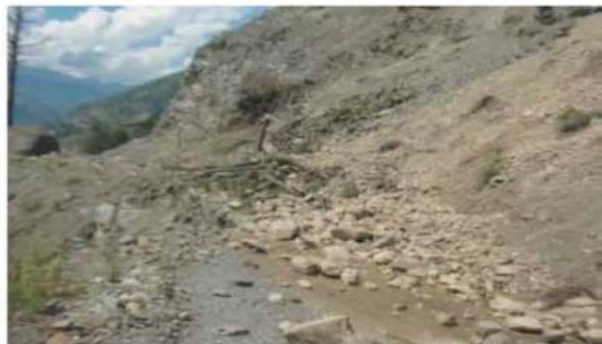
Figure 17. Photo: Condition of project approach road at different locations during rainfall.
