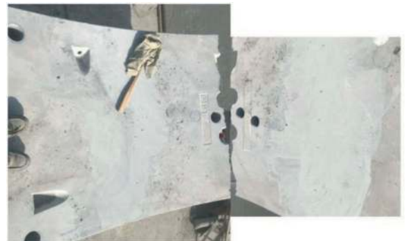
Figure 16. View of the positions where the cores were obtained for testing in one of the split SFRC segments.
