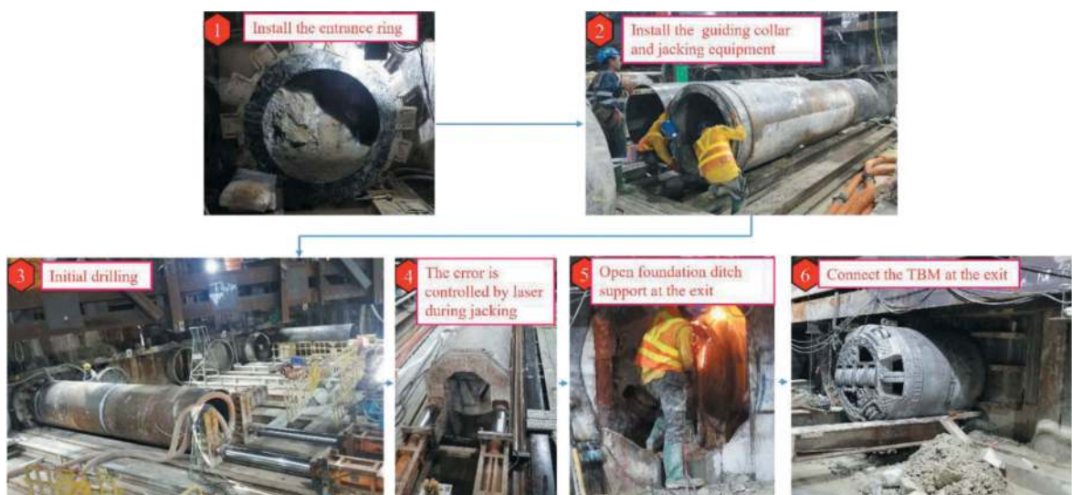
Figure 6. The procedure of the MTBM tunneling machine advanced pipe shed support technology.
