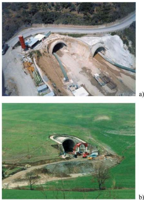
Figure 8. Examples of portal of tunnels by jet-grouting shells. (a) S.Elia Tunnel, Messina-Palermo Motorway and (b) Tunnel N2, Sibari-Cosenza Railway Line (Lunardi, 2008).
