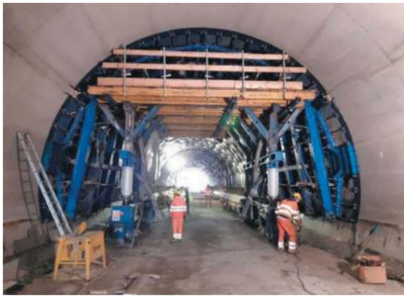
Figure 14. Relining by high strength fibre reinforced plain concrete - Pilot application at “Colle” tunnel.
