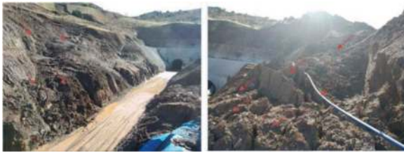
Figure 1. View of flows on the right and left slope slopes at the diversion tunnel entrance portal.
