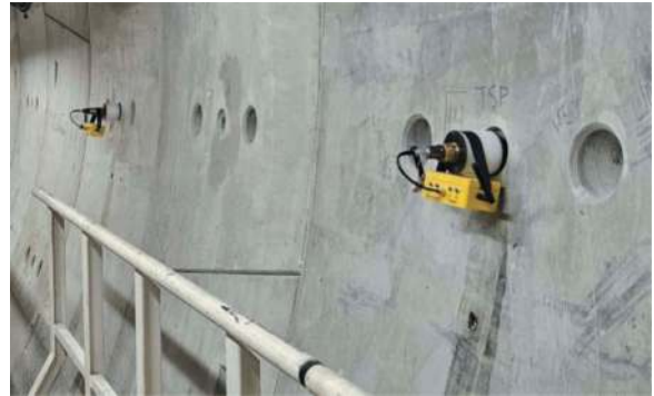
Figure 2. Two TSP 603 wireless transceivers attached to TSP receivers deployed 1.5 m deep in boreholes through the grout hole of precast segments.
