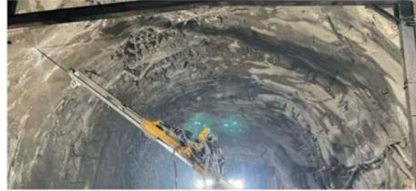
c) Steel arch buckling
