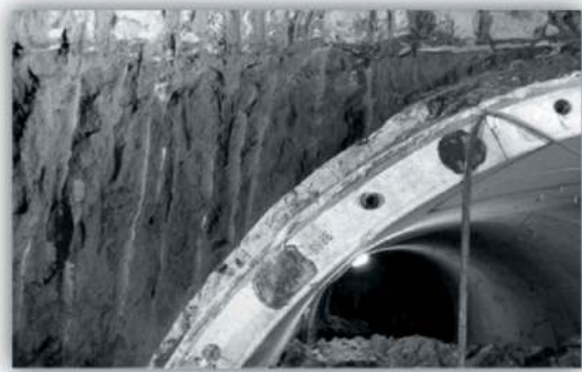
Figure 1. Backfill grouting in TBM tunnelling (gulermak umraniye goztepe metro method of statement).
