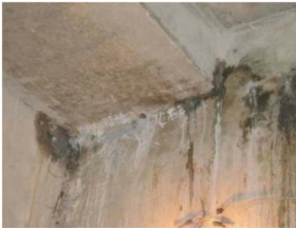
Figure 2. Example of water penetration in a monolithic reinforced concrete tunnel lining in the case of open works without backfill slots and with waterproofing based on traditional technological schemes and materials of adhesive fixing to the concrete foundation.
