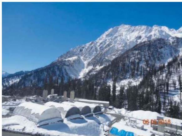
Figure 3. Rohtang's construction site at the South portal – more than 3000 m above the see.
