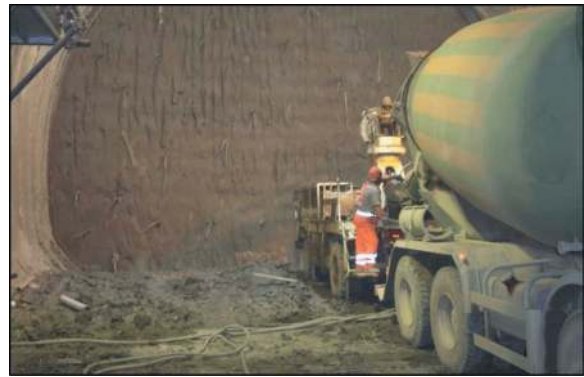
Figure 10. Furniture of the HPFRSCC at the tunnel face, ready-to-use, by means of concrete-mixer truck, is today possible.
