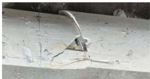
Figure 5. Damage of tunnel structure.
