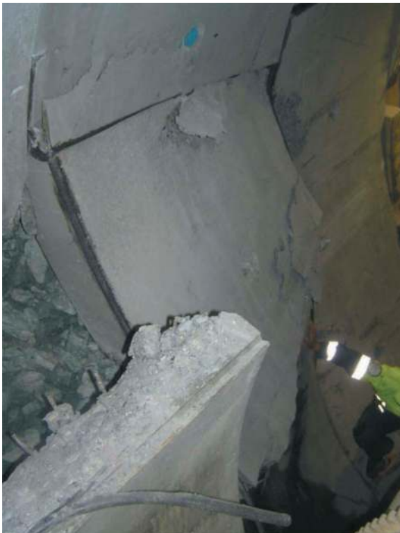
Figure 3. Damaged and shifted precast concrete segments.
