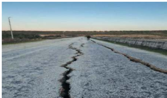
Figure 11. Primary cracks on the crest.
