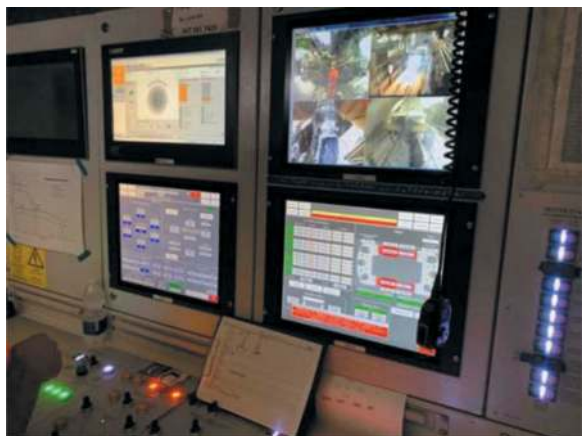
Figure 15. TPC command and control screen of the TBM in the Mules 2-3 lot.
