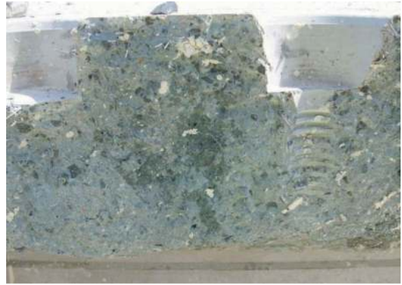
Figure 14. View of the other half of the SFRC split segment shown above, seen from the lifting sockets.
