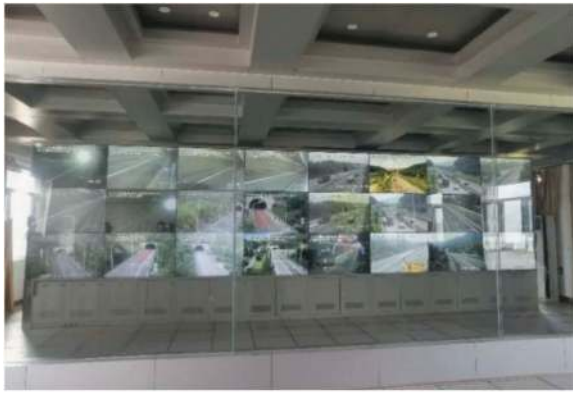
(a) monitoring center
