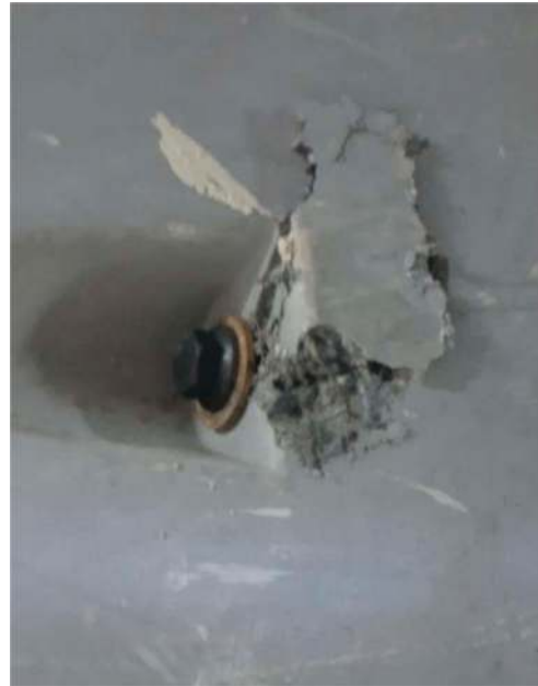
Figure 10. Pocket side-face blowout after installation of the bolt.
