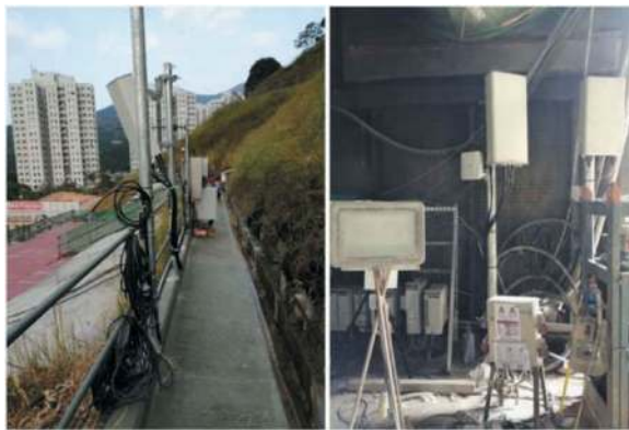
Figure 13. First On-site 5G Station (Outside/inside Caverns).
