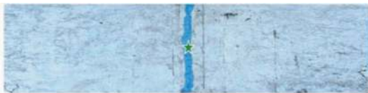
Figure 14. The crack detection result by SAM on the unwrapped image.
