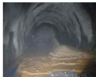
Figure 4. Sudden water inrush in the tunnel.
