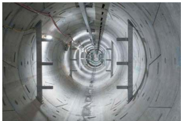
Figure 5. Example of completed tunnel lining with cable brackets installed.
