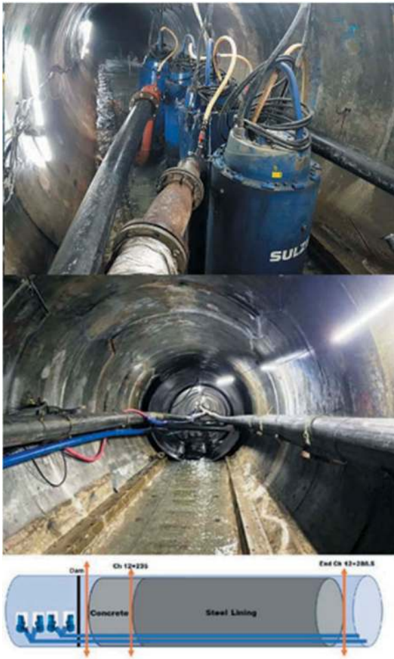
Figure 7. Dewatering sump and lines.
