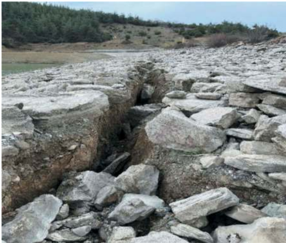
Figure 6. Openings in the upstream riprap.
