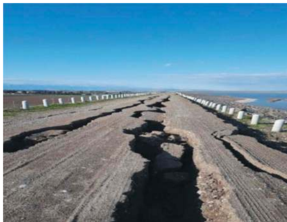
Figure 12 . Deep cracks on the dam crest.
