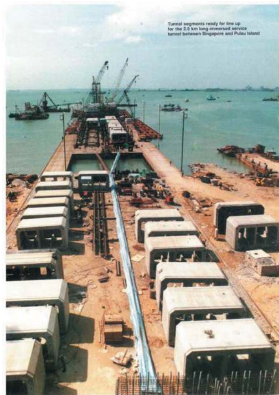
Figure 12. Singapore cable tunnel.
