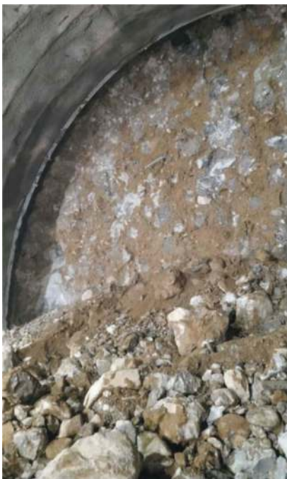
Figure 13. Section C1: detail of sub-horizontal jet-grouting column and detail of the excavated ground.
