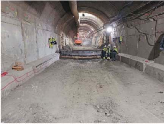
Figure 19. Refining the excavation of the inverted vault bed assist with a stencil.
