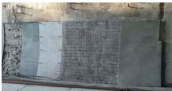
Figure 8. Experimental stand. Arrangement of the 'pie' of composite waterproof load-bearing 'diaphragm wall' at the stage-by-stage construction of two-layer concrete structure of 'sandwich' type with a middle waterproofing layer with double-sided adhesion: from left to right – model of trench 'diaphragm wall'; levelling layer with anchor releases; sprayed waterproofing layer with double-sided adhesion; reinforcing mesh, sprayed concrete layer.
