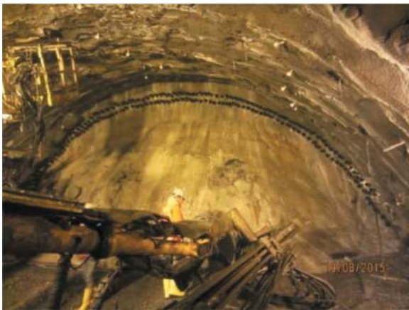
Figure 5. Installation of double pipe roof umbrella with dia 114 mm at the stretch of 2+413 to 2+445.
