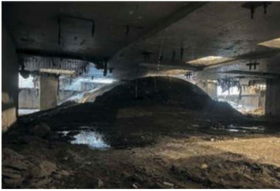
Figure 5. Polesie station crossing: general overview of the TBM, in situ soil and concrete walls.
