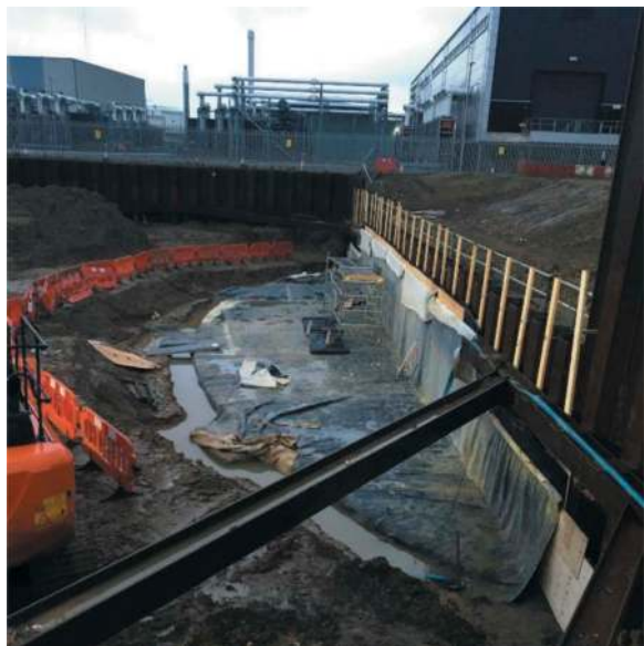
Figure 2. Enabling works cofferdam showing gasholder footprint prior to casting the protective capping slab (JSM Group, 2020).
