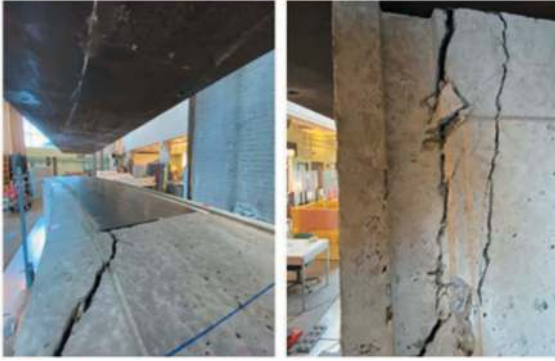
Figure 5. (a) Leading edge where radial bursting stress induced cracking is clear; (b) side of the segment where radial bursting stresses (left to right) exceeded the tensile capacity of the SFRC.
