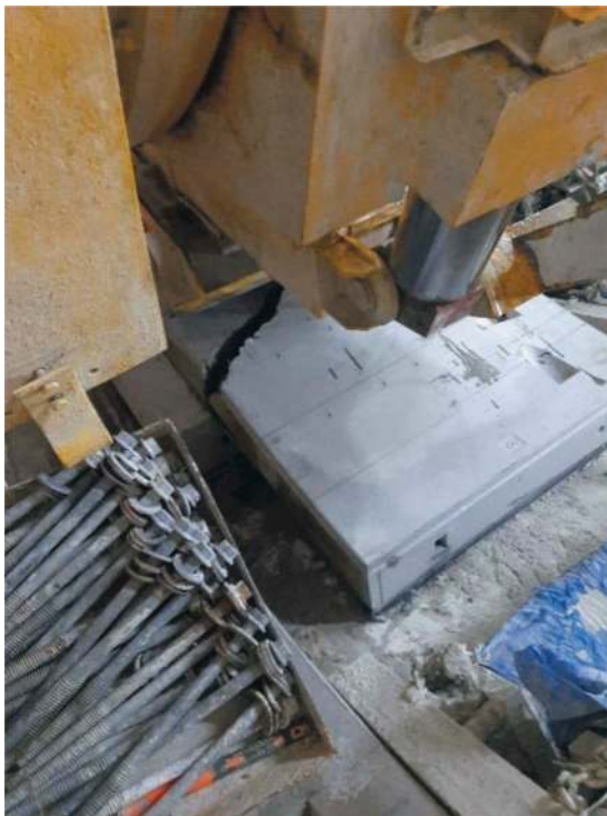
Figure 6. A different view of the broken segment shown in the previous figure.
