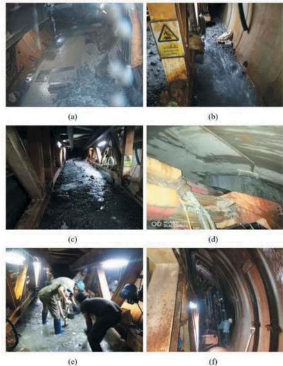
Figure 12. The major stoppage (i.e., the 1st incidence of the collapsed segment) (a) collapse occurred (b) water inflows into the tunnel (c) inrush materials with water inflows (d) the collapsed segments (e) cleaning the inrush materials (f) support tunnel with H-beam steel arch.
