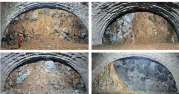
Figure 7. Different locations where mixed face support was applied in the same tunnel. Source: Authors.
