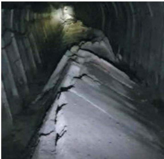
Figure 10. Heave of the bottom shotcrete support.
