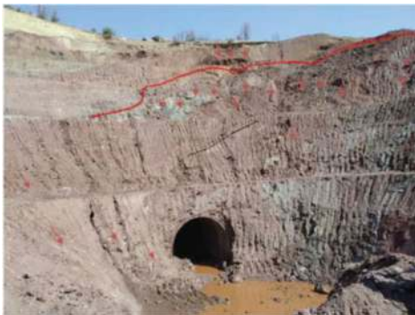
Figure 2. View of the diversion tunnel exit portal and slope failure.
