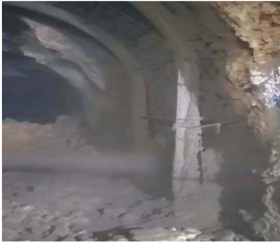
Figure 8. Deformed steel ribs on the side wall.
