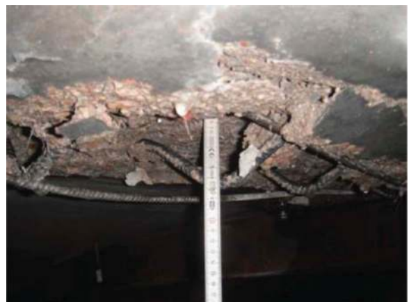
Figure 6. Failure of a segment in tunnel 26.
