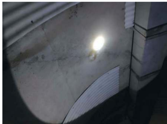
Figure 4. Minor cracks observed in the lining.
