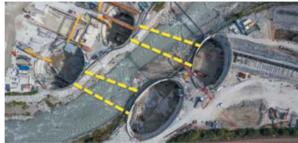
Figure 5. View from above of the 4 large shafts on the banks of the Isarco River.
