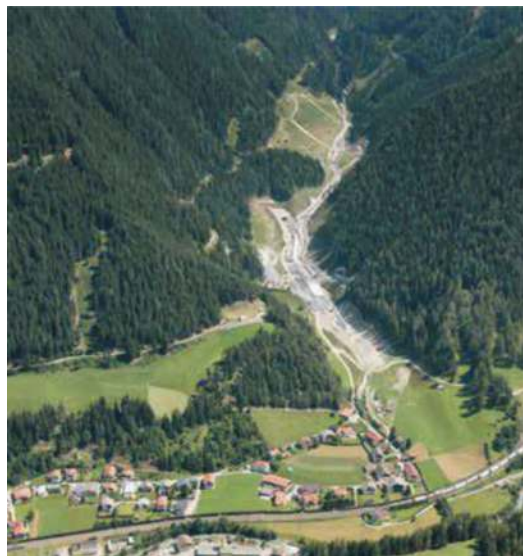
Figure 7. View of the Padaster valley spoil disposal site at the beginning of construction.
