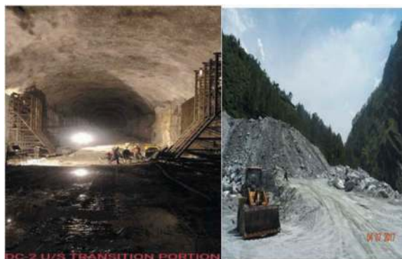
Figure 12. Shows the shutters used on both sides of Desilting chamber and view of dumping yard.
