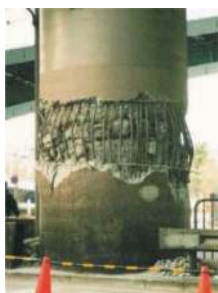
Figure 23. Seismic damage (Hanshin Expressway Management Engineering Center et al., 2020).
