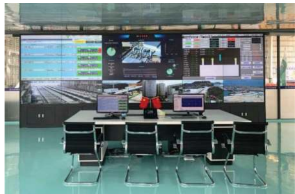
Figure 5. System control room.
