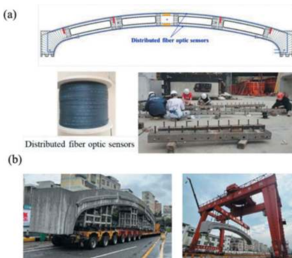
Figure 3. Application of distributed fiber optic sensors for monitoring large scale prefabricated structures inside subway station (a) position and installation of distributed fiber optic sensors, and (b) transportation and assembling process of vault structures.
