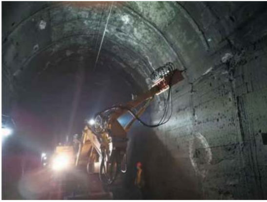
Figure 12. Chipping operation of the complete equipment for treating the defects of operating tunnels.
