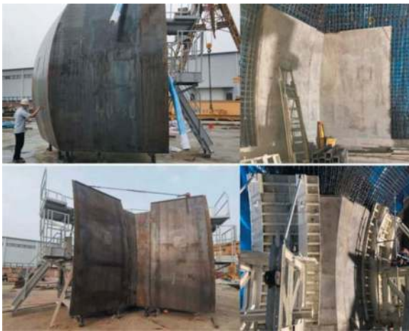
Figure 14. Sidewall formwork reconfigured in inner (top) and outer (bottom) corners using insert pieces.
