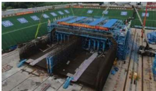
Figure 30. Full-section casting formwork of Chebei-Xinjiao West Road tunnel (source: CCCC4th Harbor Engineering Co. Ltd).
