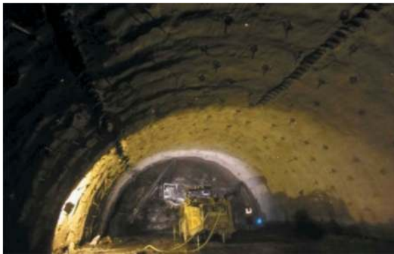
Figure 7. Two rows of LSC, then 1 row of LSC close to tunnel face of top heading, NP at July of 2015.
