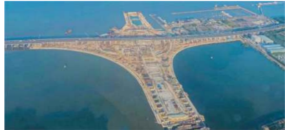
Figure 3. Bird's-eye view of construction of the East Artificial Island and tunnel excavation.
