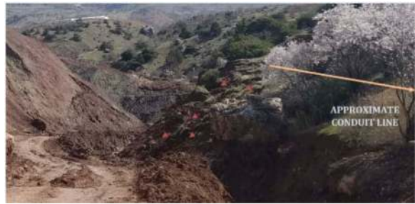
Figure 4. View from the slides on the hillside at diversion tunnel outlet conduit route.
