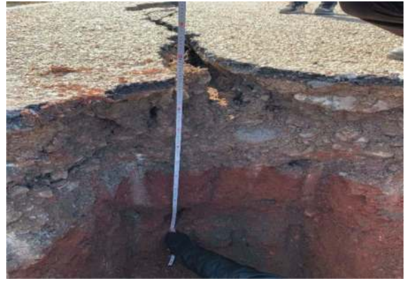
Figure 16. Longitudinal cracks and subsidence on the dam crest.
