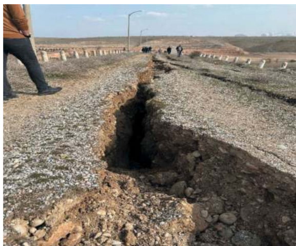
Figure 3. Cracks along the dam crest.
