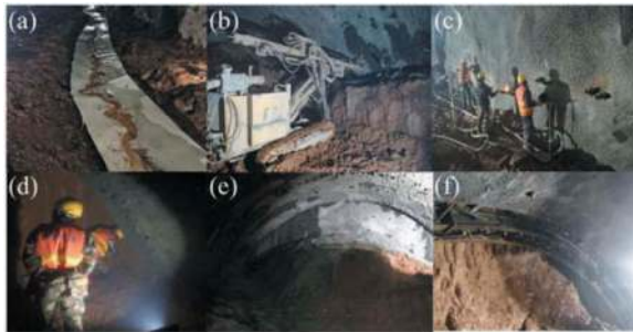
Figure 11. Site control countermeasures (a: arch foot drainage ditch; b, c: application of foot-lock bolt; d: application of large arch foot; e: seal of tunnel face; f: advance pipe shed and small pipe grouting).
