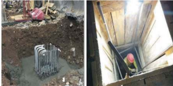
Figure 9. Aspect of a final hand excavated squared pile and a moment of its construction.
