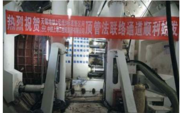
Figure 13. Launching of the pipe jacking machine in the cross passage of Wuxi Metro Line 3.
