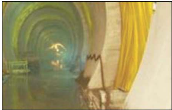
Figure 3. Construction of a complete tunnel lining consisting from right of: spritz-beton, a waterproof plastic membrane and a cast-in-place concrete final lining.
