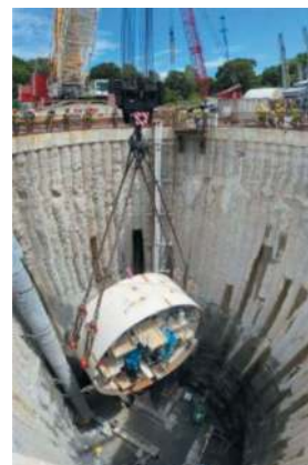
Figure 9. 375 tons TBM front shield lowered with the 600 tons crawler crane in the launch shaft.
