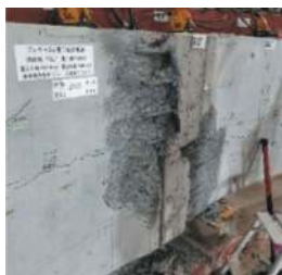
Figure 14. Condition of the main reinforcement failure.
