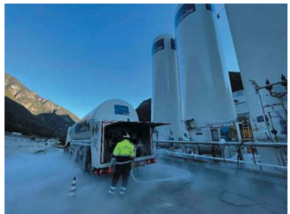
Figure 9. Liquid nitrogen supply to the storage facility.
