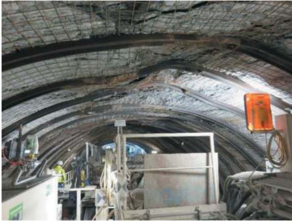
Figure 10. Deformation of the steel profiles in the top heading.
