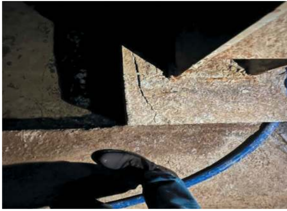
Figure 14. Cracks in the penstock support concrete.
