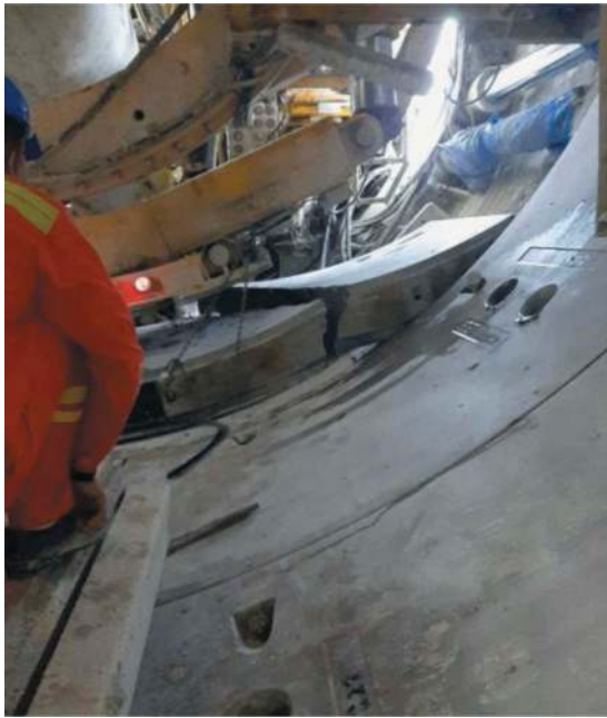
Figure 5. SFRC segment broken during ring assembly.
