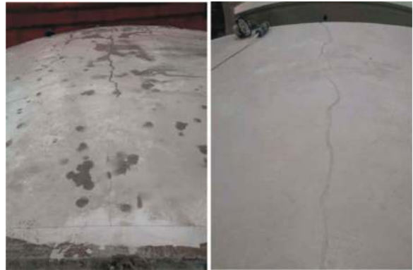
Figure 4. Detail of crack traversing the entire segment face before and after repair.
