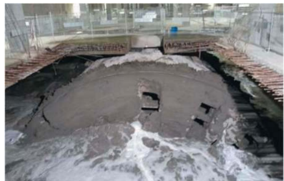
Figure 4. Polesie station crossing: the TBM advances with limited gap on the top.
