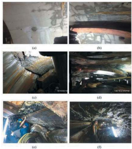
Figure 15. The major stoppage (a) segmental lining cracking (b) cluster cracks of the collapsed segments (c) damage of the segmental lining (d) the collapsed segments (e) H-beam steel rib used for supporting the problematic zone (f) inspection and working for support the ground.
