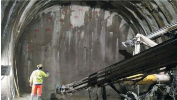
Figure 15. Creation of sub horizontal columns of improved ground under the tunnel floor.
