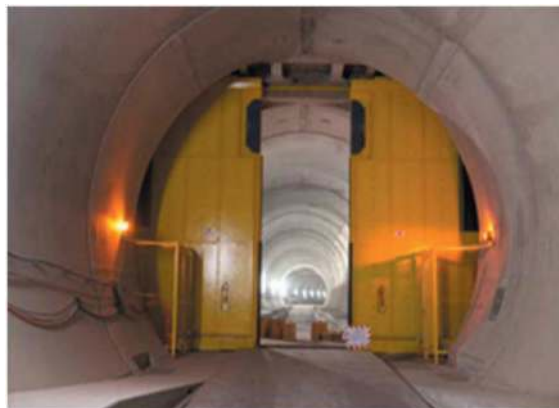
Figure 3. Fire Door within Crossover Tracks of the Gotthard Base Tunnel.
