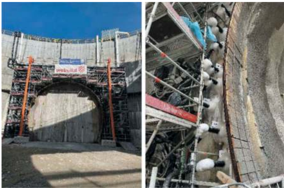
Figure 7. View of the GNBDI south portal and detail of the freezing probes.
