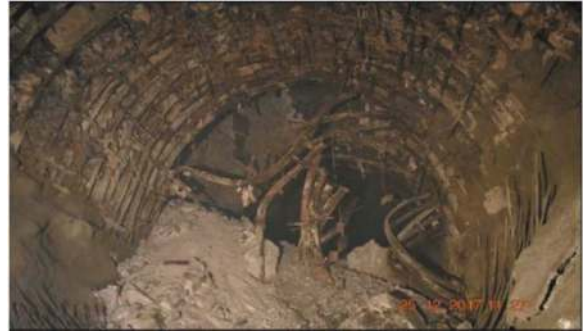
Figure 10. Distortion of high-capacity tunnel.
