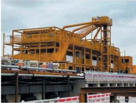
Figure 3. The slurry separation equipment.
