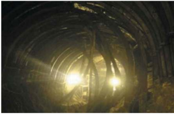
Figure 8. Dislodging of Steel Ribs at Shear Zone.
