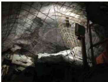
Figure 3. Damage of bracing system caused by rock burst.
