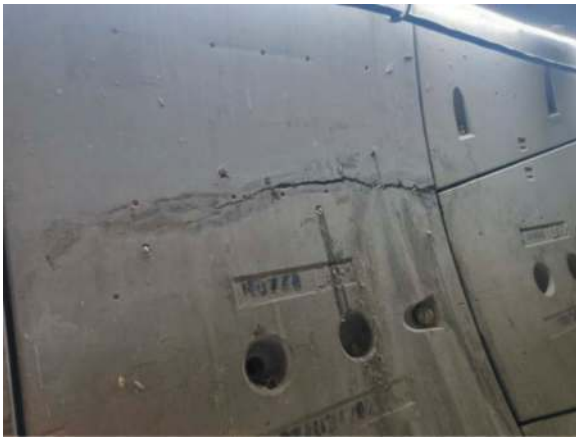
Figure 8. Crack during the installation of the next ring segments due to the thrust of the TBM jacks.
