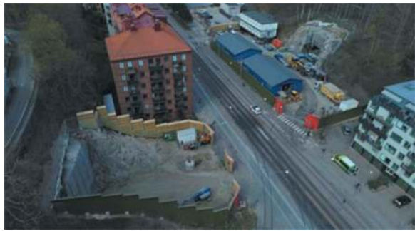
Figure 10. Portals and site installation area of service tunnels 206 (left) and 207 (right), access to Lorensberg and Liseberg.
