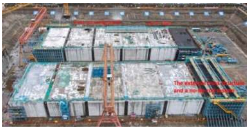
Figure 29. Full-section casted elements with post-pouring band in between (source: CCCC4th Harbor Engineering Co. Ltd).
