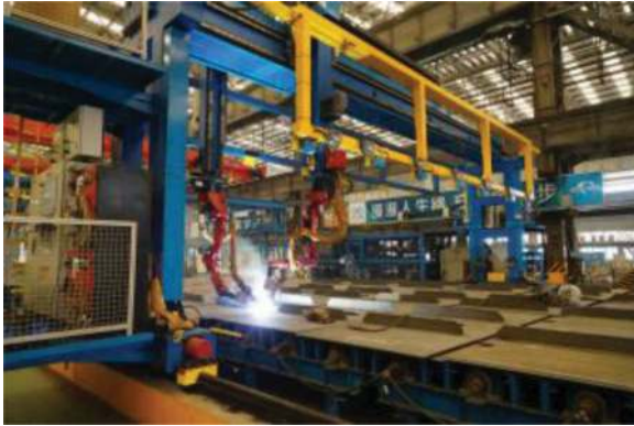
Figure 4. Intelligent welding line.
