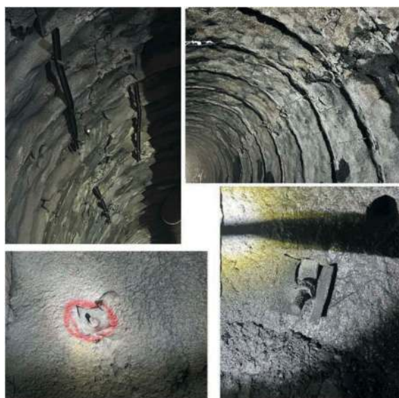
Figure 3. Rock support defects due to low squeezing.
