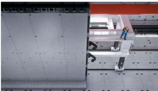
Figure 14. Grabbing pin shaft separated from the Mid-partition.
