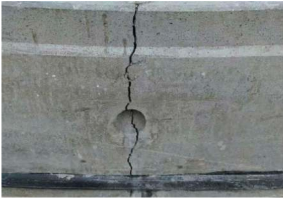
Figure 12. A view of the crack above, across the face of the circumferential joint.
