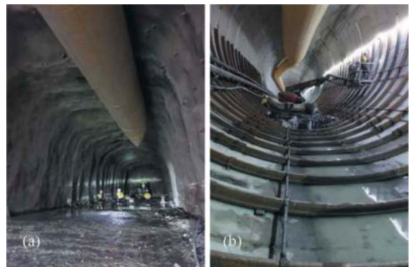
Figure 17. Central Heading Tunnel excavated in MH (a); Sliding steel rib installation in MAT01 (b).
