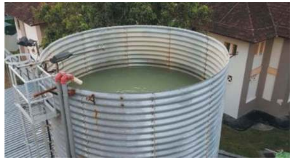
Figure 6. Slurry treatment plant active tank.
