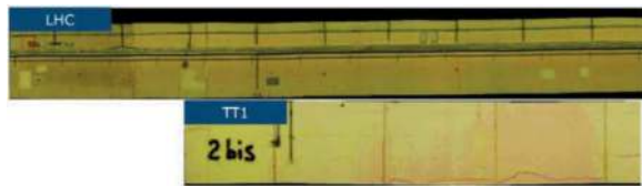
Figure 6. Crack spatial layout after the detection.
