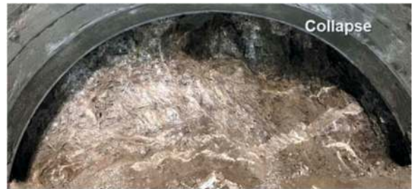
Figure 9. Collapse occurred to ~2.0 m depth within the weak layer in the diagonal tunnel.
