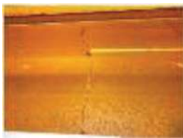
Figure 2. Crack of road pavement caused by ground heave.
