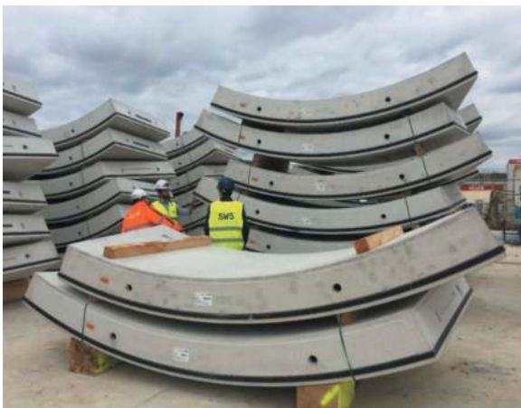
Figure 9. GP M14 Lot 4 precast lining: segments delivered on site (left) and Koumba TBM ready for launching (right).
