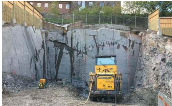
Figure 11. Abutment walls of access tunnel 206 with the Carlanderska Hospital in the background.
