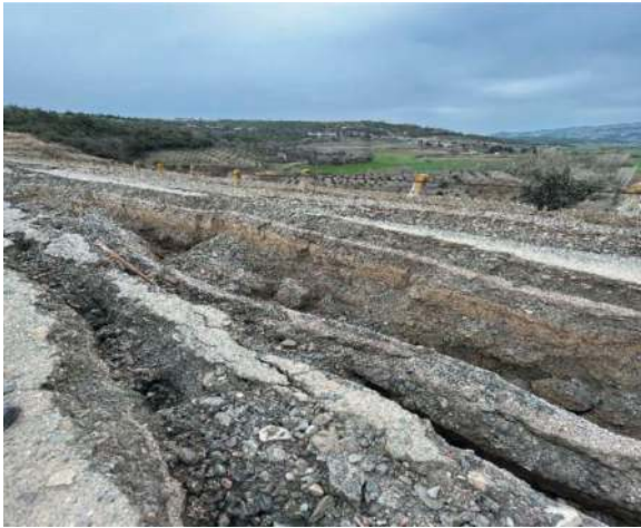
Figure 5. Wide-span splits along the dam crest.
