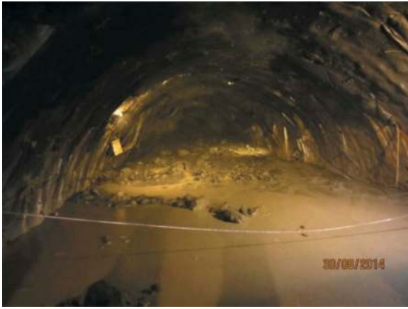
Figure 4. Material wash out at top heading in ch. 2+390 dated 30/08/2014.
