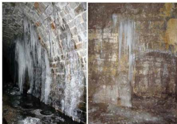
Figure 1. Water seepage through cracks in the lining.
