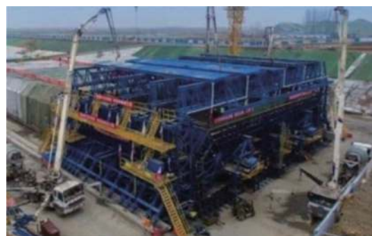
Figure 28. Full-section casting and prefabrication with integral hydraulic formwork of Xiangyang- Hanjiang Tunnel (WANG Yong, et al.2022).
