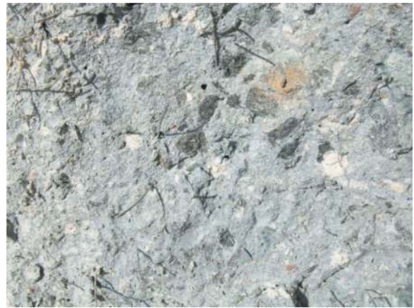
Figure 15. Detail of the concrete mass with fibres from the same splitting surface.
