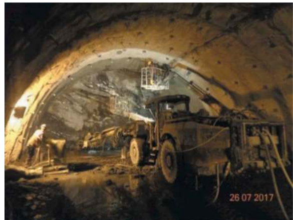
Figure 6. One row of slot in the primary lining behind tunnel face of the top heading, NP at July of 2017.
