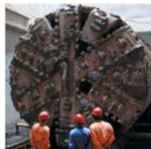
Figure 10. Cutter head of shield machine in Hua-Guang section of Guangzhou Metro Line 9.
