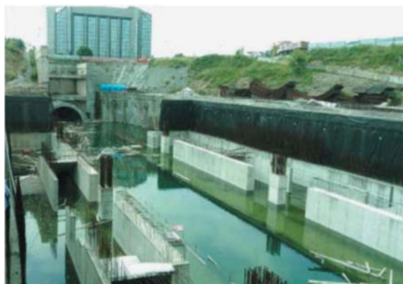
Figure 3. Flooding of the executed works.
