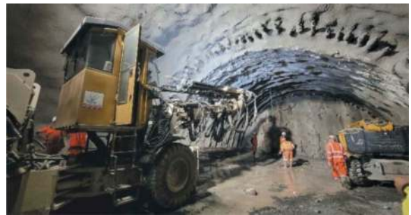
Figure 12. Excavation works for technical cavern where the first TBM will be assembled.
