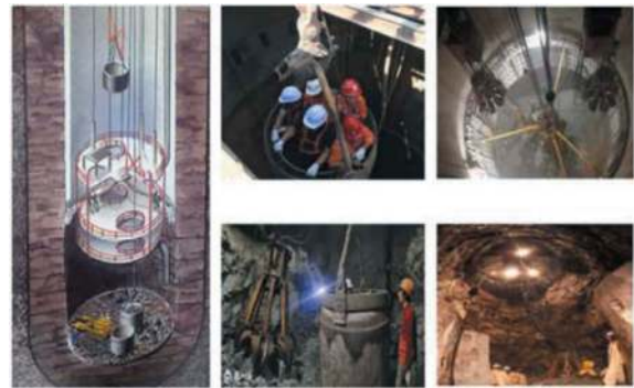
Figure 1. Main device and equipment configuration of drilling and blasting well construction system.
