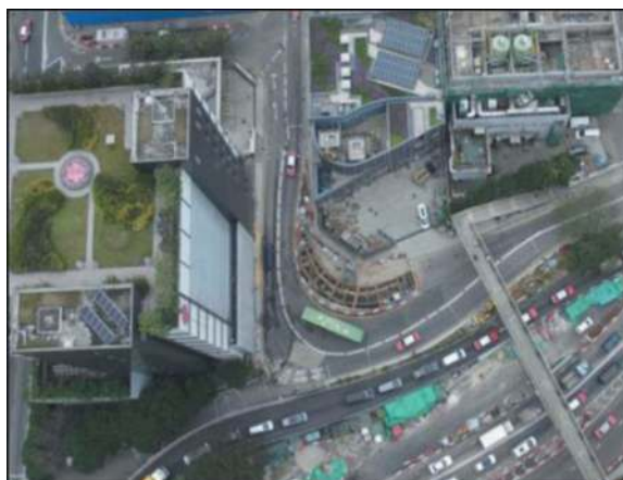
Figure 7. Traffic management and temporary trenching for sheetpile removal at Wan Shing Street.
