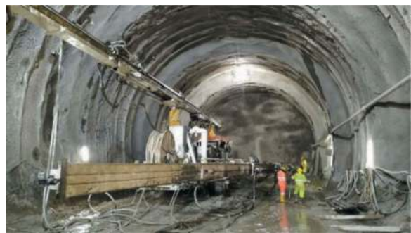
Figure 14. Reinforcement of the core-face with sub horizontal columns of ground improved by means of jet-grouting.
