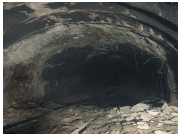
Figure 7. Disintegration of shotcrete and wiremesh.
