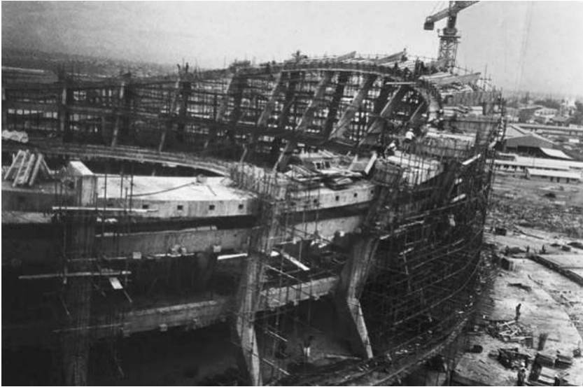
FIGURE 34. National Theatre in Lagos, construction in progress. Source: TsDA, f. 608, op. 6P, a.e. 6, Technoexportstroy catalog.
