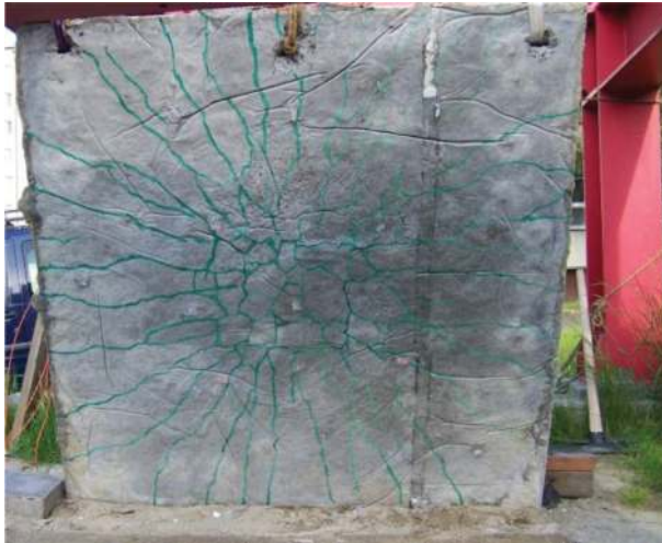
Figure 6. Cracks on the bottom surface of the slab.
