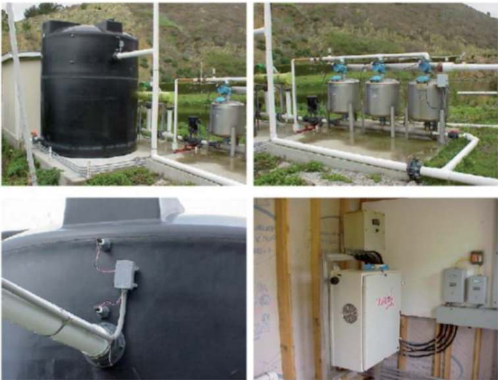
Figure 2. Ozonated water in the irrigation system.
