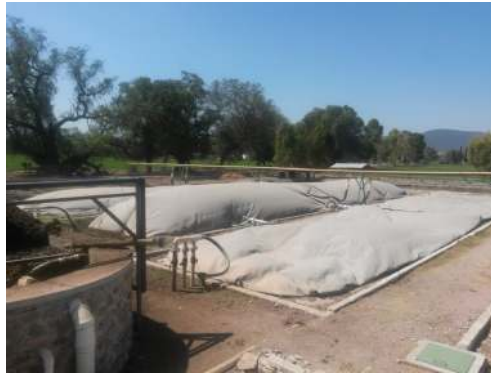
Figure 2. Covered lagoon digesters for cow manure treatment.
