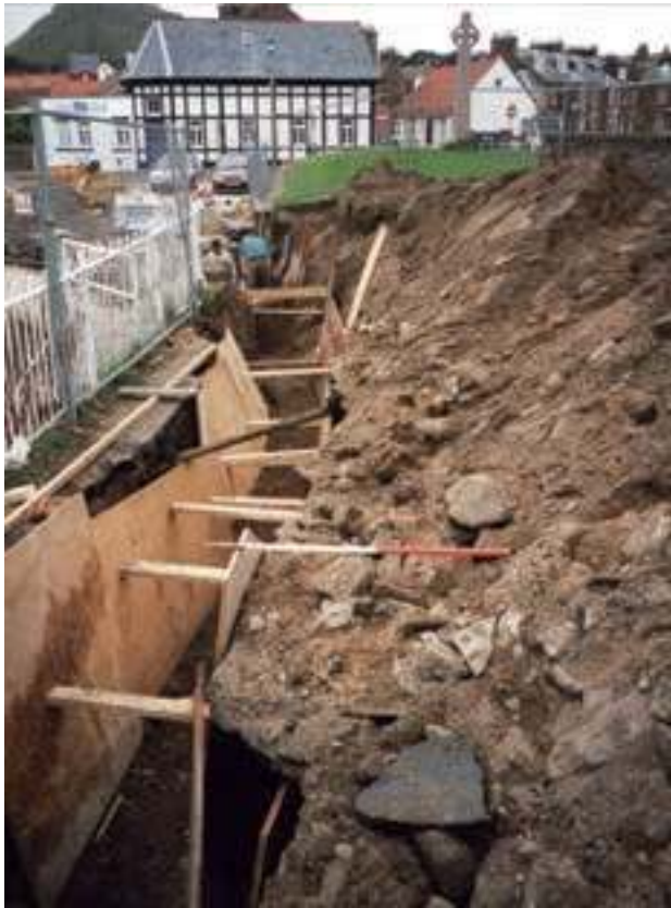
Fig. 1.9: General excavation of the services trench behind the sea wall (trench 5), looking south
