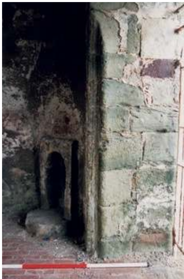
Fig. 4.27: The western jamb of the south entrance to the church preserved within the upstanding porch (note the fireplace and chimney breast above, inserted in the 19th century)
