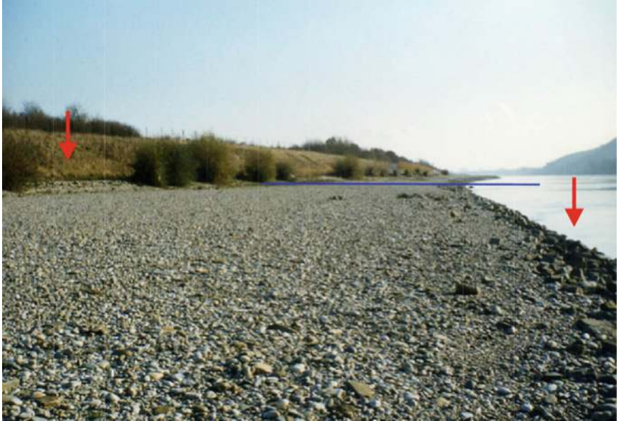
Fig. 24.5 Extended underwater gravel bank inshore structure under construction; red arrows indicate “double riprap”; blue line indicates the water level nowadays after construction (Section 2)
