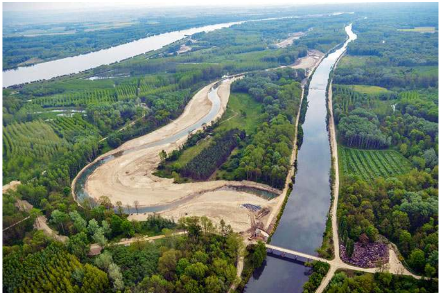
Fig. 15.4 Bifurcation of the newly excavated riverbed with the adjoining lowered floodplain terrain (left) from the old straight Traisen canal (right) prior to its flooding (in the background: Danube River; source: M. Haslinger and Verbund AG 2014)
