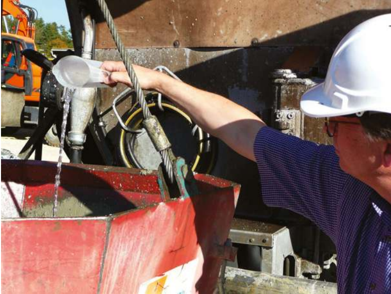
FIGURE 5.3 Intervention A. Work in progress. Adding mineralwater to all waterbased materials used for the construction of the building.
