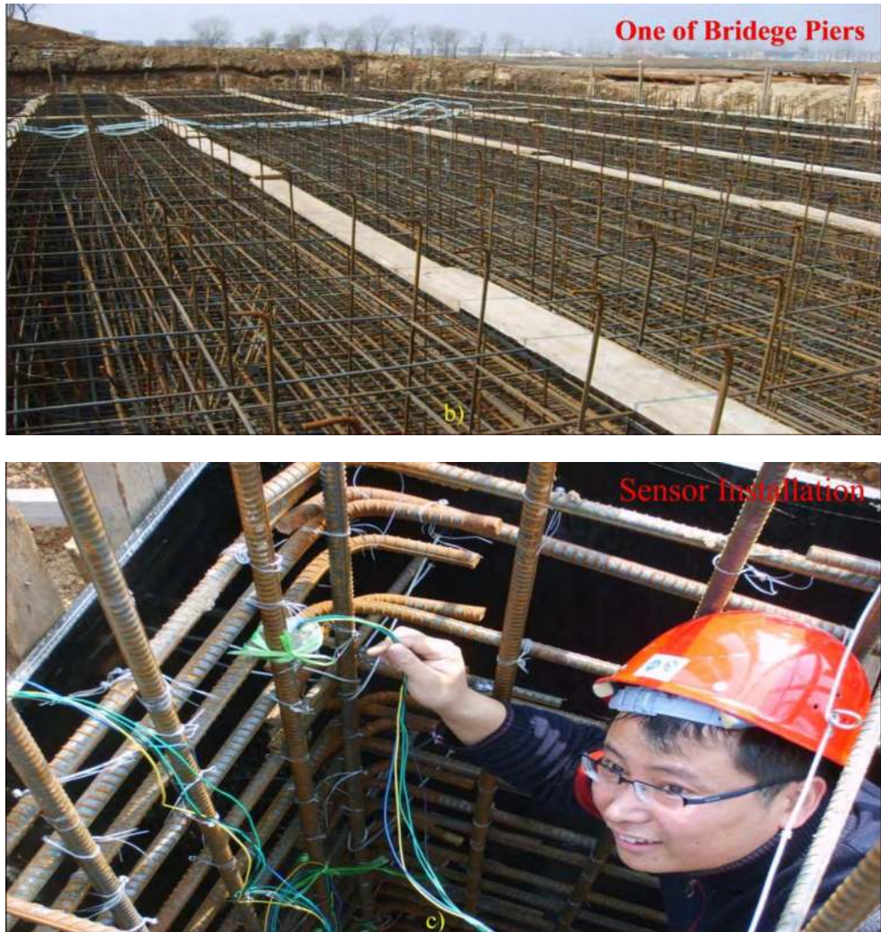
Fig. 32. Corrosion monitoring of the bridge pier. Scheme of the sensors' location a), Bird's eye view of the pier b) , and the sensor installation c)
