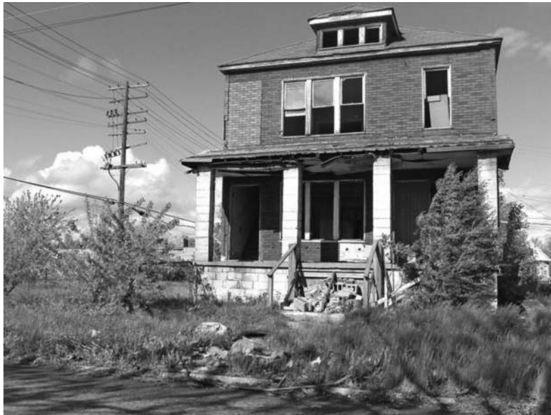
Figure 1.5 Thousands of Abandoned Houses in Detroit. Detroit has hemorrhaged population and has no hope of regaining its former size. The photograph reveals not only a vacant structure but also vacant lots where housing once stood. Detroit no longer needs the extensive housing stock that once provided shelter for the city's peak population. As a result, Detroit, like other "shrinking cities," initiated extensive efforts to raze abandoned houses and properties suffering advanced disrepair.
