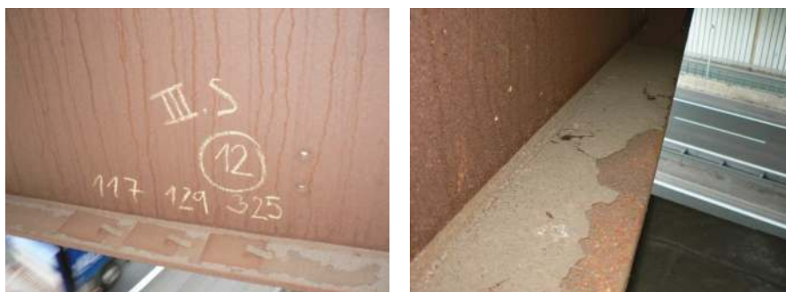
Figure 8. Bridge No. 1—unfavorable development of corrosion products on the internal upper surface of the bottom flange (surface P6).
