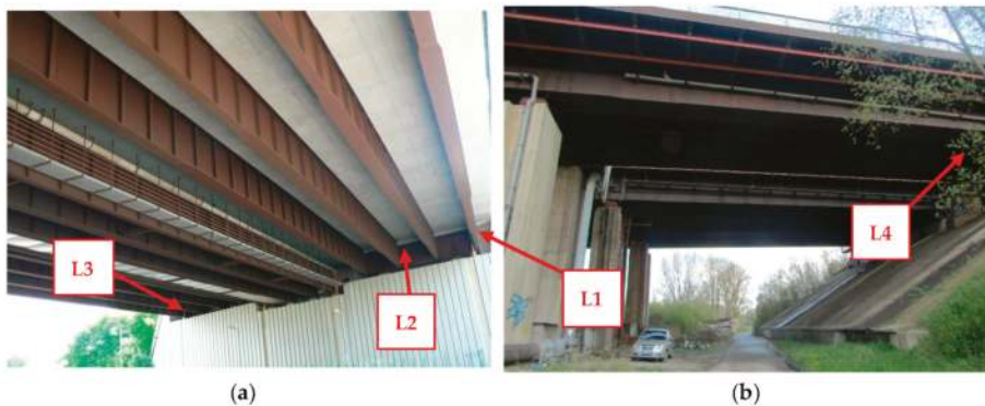
Figure 6. Position of the measuring devices on the selected bridge structures—bridge No. 1 (a) and bridge No. 2 (b).
