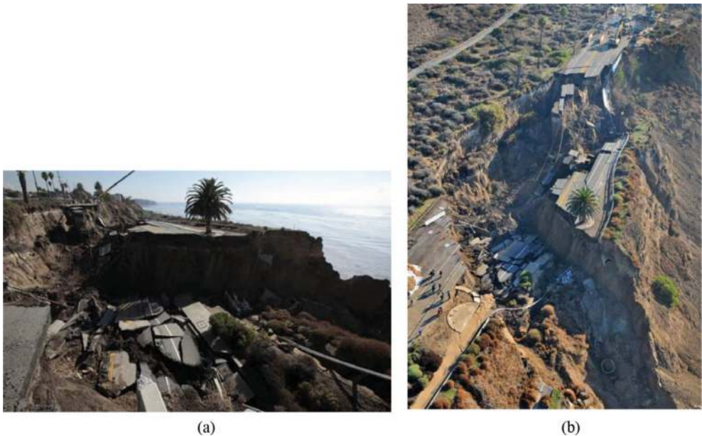
Figure 11. (a) The collapse of the highway in California and (b) view from airplane.
