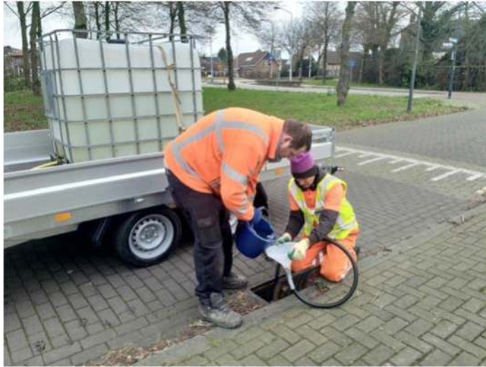
Figure 6.17 Pouring cold water onto the cable, in the underground sewer, using a hose and a funnel for validation of the measured distances by the DTS system. Source: courtesy Remy Schilperoort (Partners4UrbanWater).
