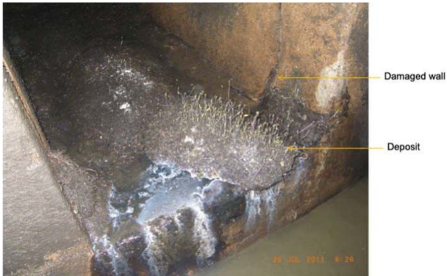
Figure 3.3 A sewer section where sediment deposit and damaged wall hinder installation of sensors for discharge measurement. Source: Université Gustave Eiffel.
