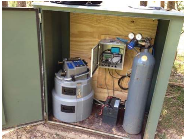
Figure 7.7 Metal cabinet housing monitoring devices. Source: Peter Poelsma (University of Melbourne).
