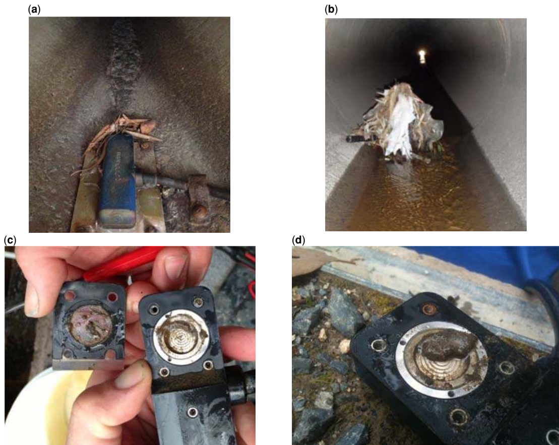
Figure 4.3 Debris caught on sensors blocking sensor beams (a, b), sediment on diaphragm of a pressure sensor (c, d). Source: Peter Poelsma, University of Melbourne.
