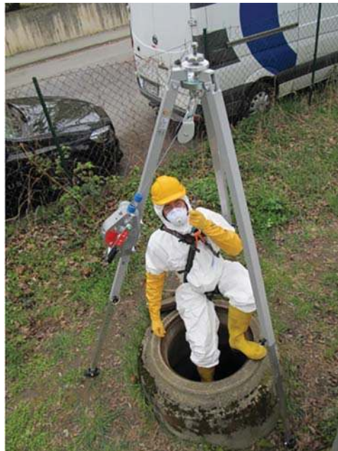
Figure 7.4 Entering the sewer network with a tripod. Source: Jakob Benisch (TU Dresden).
