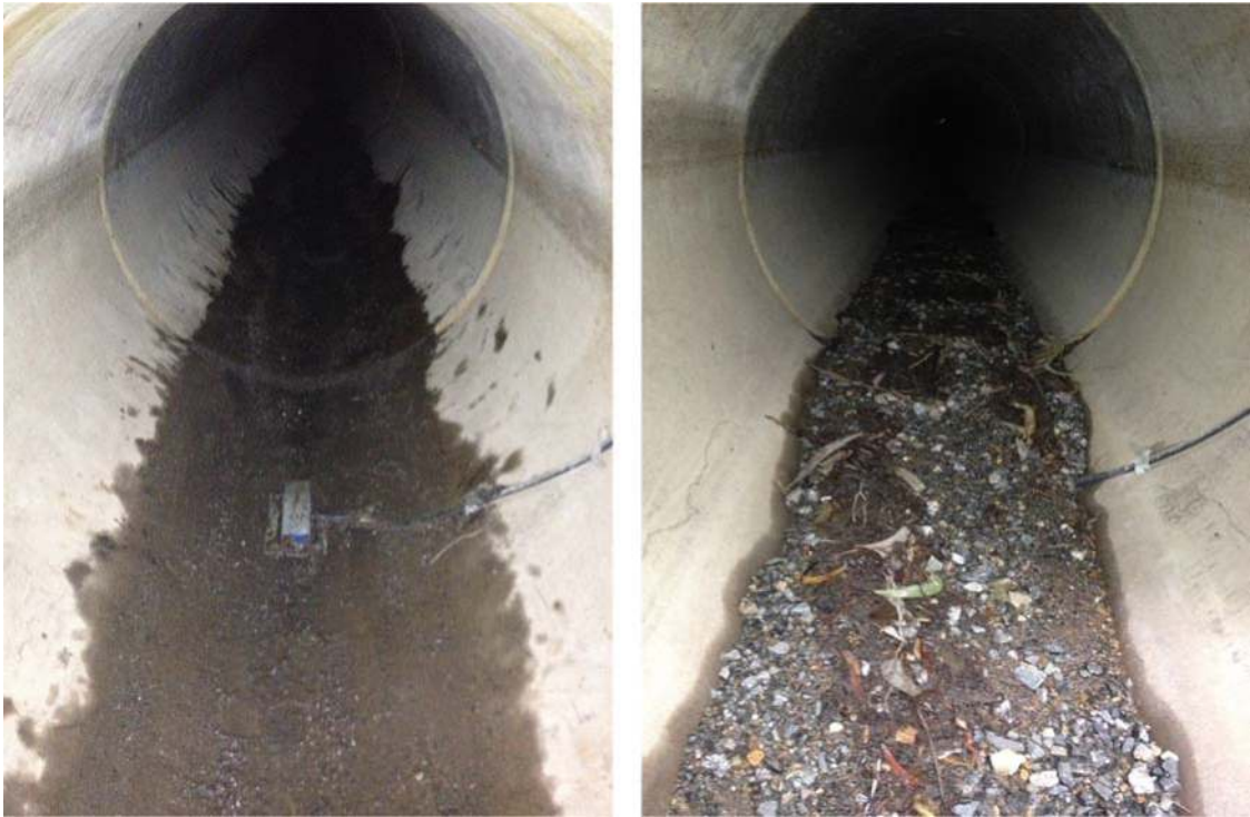
Figure 4.4 Example of a flowmeter being covered by sediments after a storm event, leading to loss of reliable data. In this case sediment accumulation was due to the construction of a small weir downslope of the probe. Source: Peter Poelsma (University of Melbourne).
