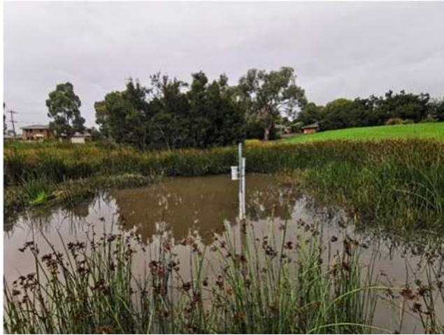
Figure 7.8 Ultrasonic (left) and capacitive (right) sensors for water level monitoring installed in PVC pipes and above the water to avoid any vandalism – wetland in Melbourne, Australia. Source: Frédéric Cherqui (INSA Lyon).
