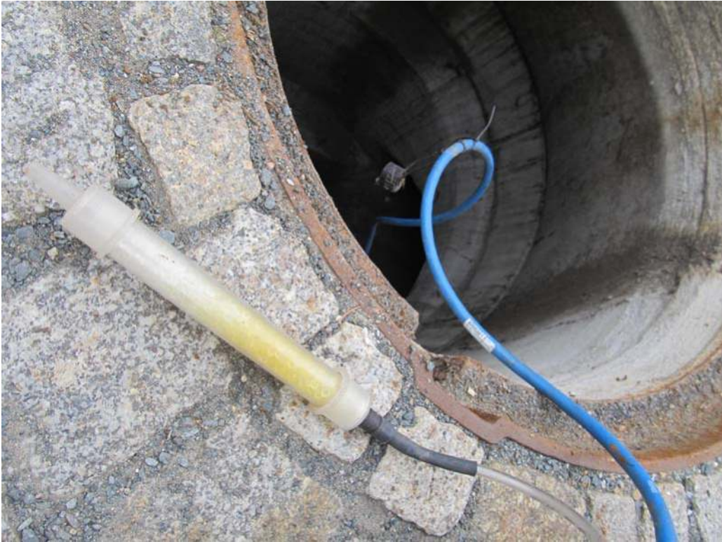
Figure 7.20 Half-used silica capsule of a water level sensor. Source: Jakob Benisch (TU Dresden).
