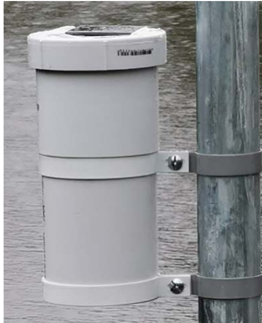
Figure 7.16 Self-powered water level monitoring system using three AA rechargeable batteries and a 0.5 W solar panel (on top). The data are sent every 15 minutes using the SigFox network – wetland in Melbourne, Australia. Source: Frédéric Cherqui (INSA Lyon).
