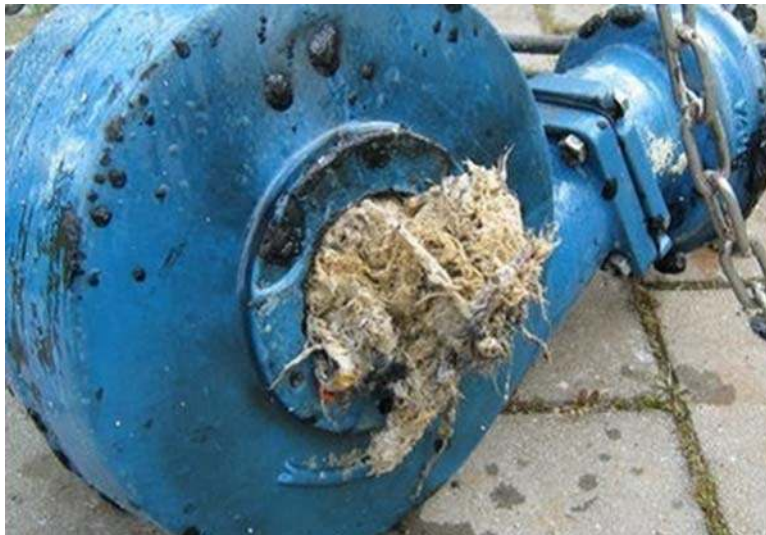
Figure 3.43 The cause of an increase in energy consumption became immediately clear when inspecting the pump. Source: courtesy Kees Kooij (Deltares).
