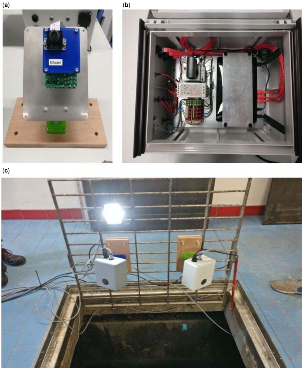
Figure 6.19 Example of cameras installed in a wastewater pumping station: (a) Camera including electronics; (b) Camera housing, (c) Two cameras installed at a grate in a wastewater pumping station. Source: courtesy Antonio Moreno-Rodenas (Deltares).
