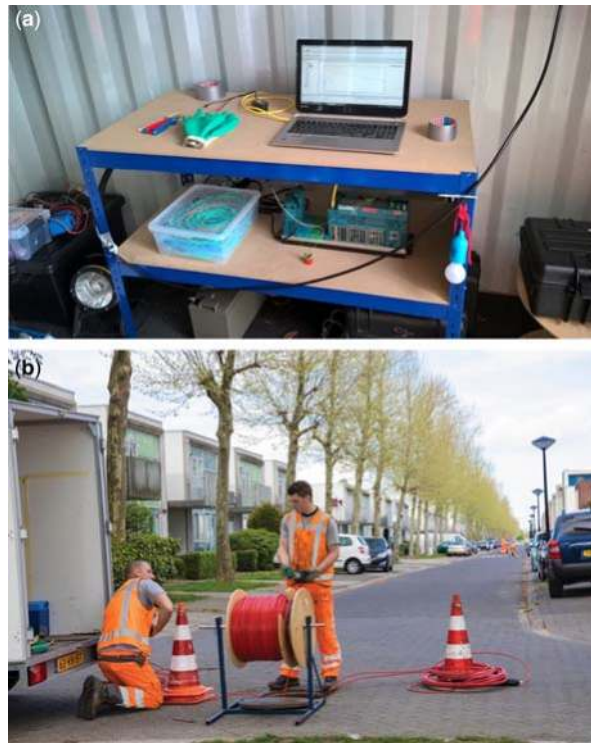
Figure 3.51 (a) DTS measuring computer, (b) Installation of a DTS cable. Source: courtesy Rémy Schilperoort (Partners4UrbanWater).
