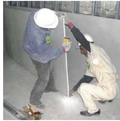
FIG. 80 The building assembly is often accompanied by in-situ adjustment work and schedule conflicts by the subcontractors working in the same space at the same time.
