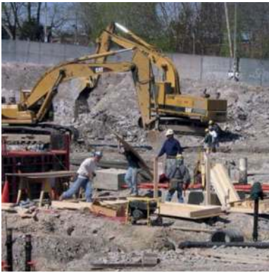
FIG. 79 The individuality of most building-sites makes them difficult to plan and often conflicts and inefficiency can be observed.
