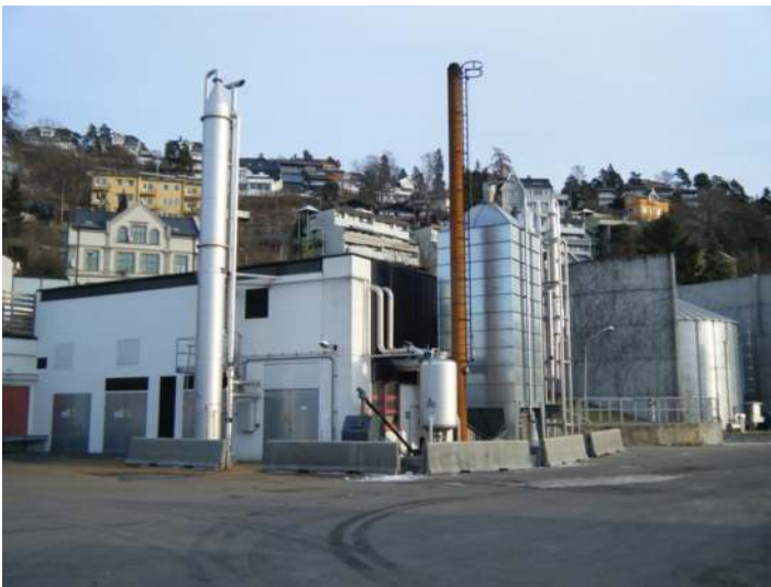
Figure 18.3 The biogas upgrading plant at Bekkelaget, Oslo (picture courtesy: Oslo Water and Wastewater Authority, Norway).
