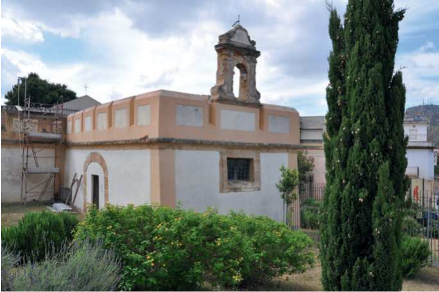
FIGURE 3.3 Oratory of Villa Cattolica, entrance from the inner garden, Bagheria (Palermo) PHOTOGRAPH BY THE AUTHOR
