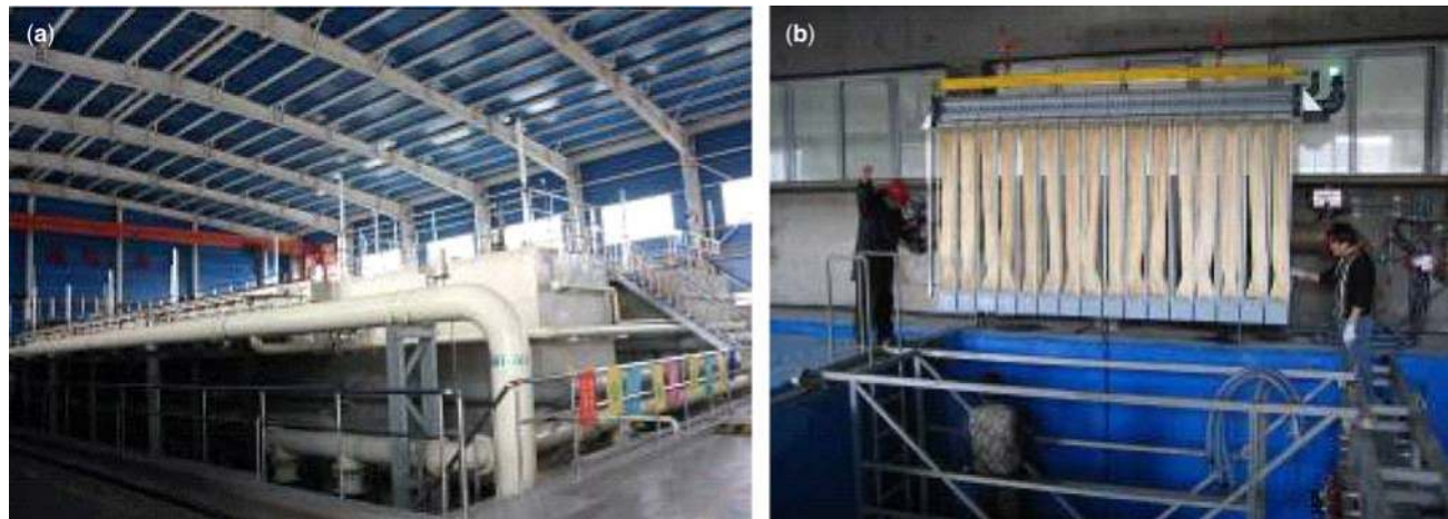
Figure 23.4 Views of the QingHe water reclamation plant (a) and the BeiXiaoHe water reclamation plant (b). (a) Tertiary filtration – ZeeWeed 1000 membrane tanks (b) MBR – installation of a Memcor Memjet module.
