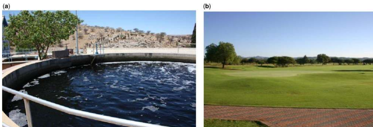
Figure 29.5 View of the Old Goreangab Water Reclamation Plant (a) and the golf course of the Windhoek Country Club (b).
