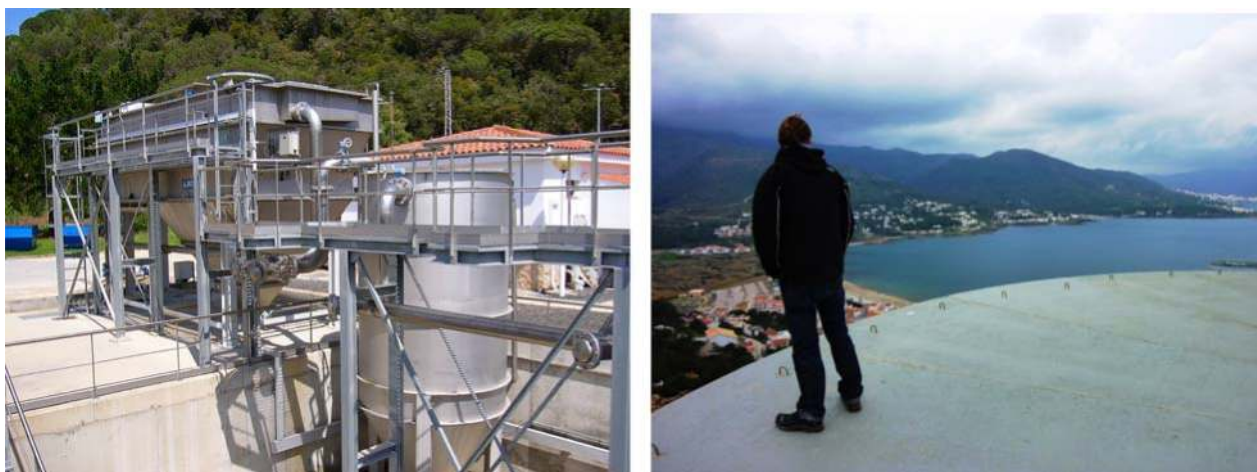
Figure 4.1 View of the tertiary treatment at Tossa de Mar and the gravity storage tank for reclaimed water in El Port de la Selva.
