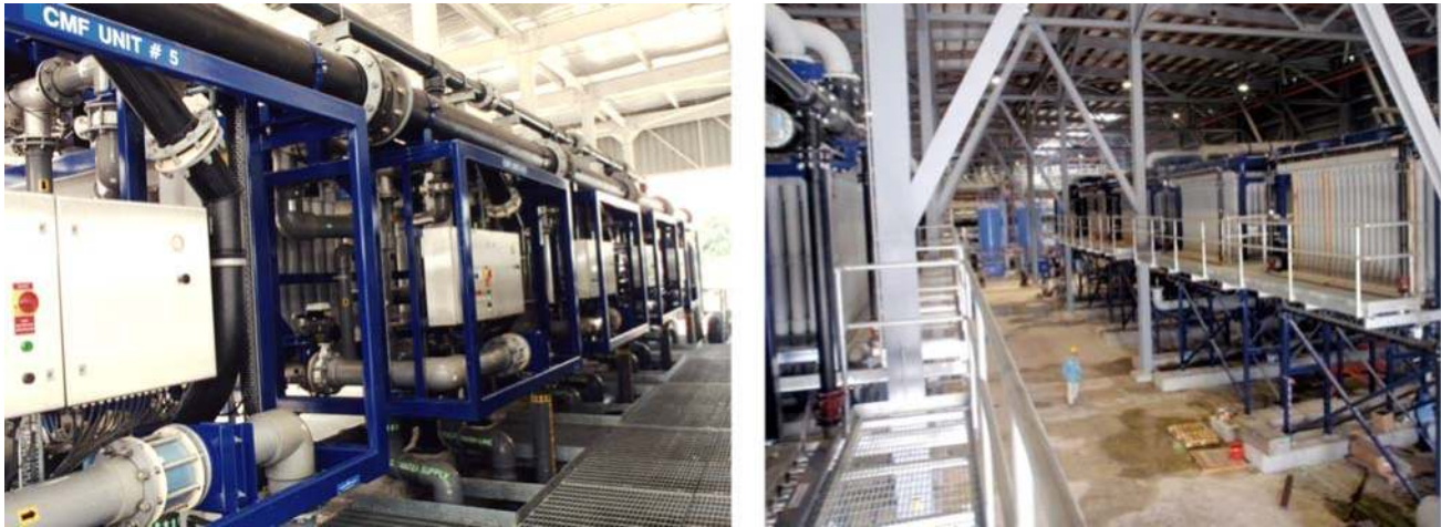
Figure 3.4 NEWater production process: view of microfiltration.
