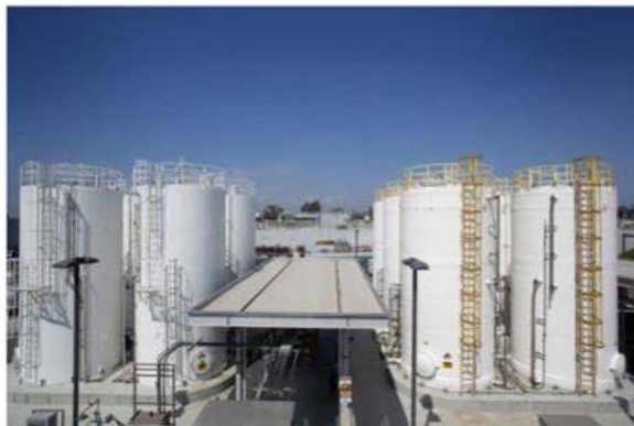
Views of the Advanced Water Purification Facility.
