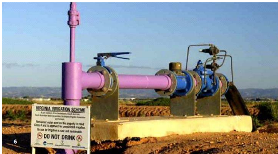
Figure 17.4 Farm connection, Virginia pipeline scheme (Photograph courtesy of Arris Pty. Ltd., Melbourne).
