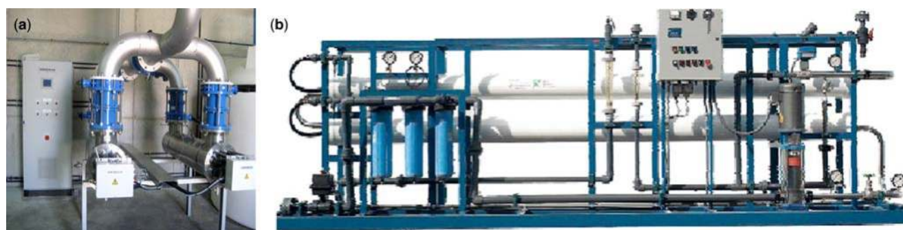
Figure 8.3 Views of UV disinfection (a) and ultrafiltration modules (b).
