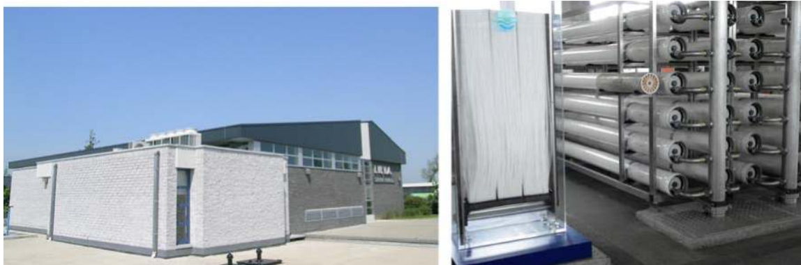
Figure 26.1 General view of the Torreele recycling facility and the membranes of ultrafiltration and reverse osmosis.
