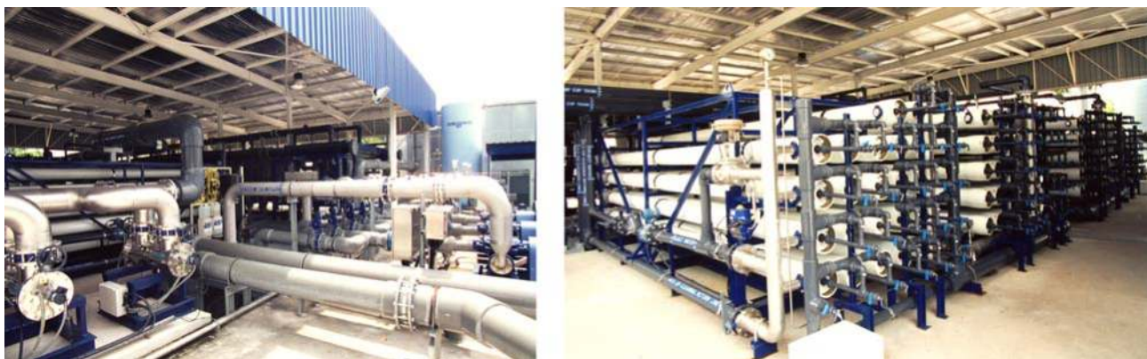
Figure 3.2 Views of the Bedok NEWater demonstration plant.
