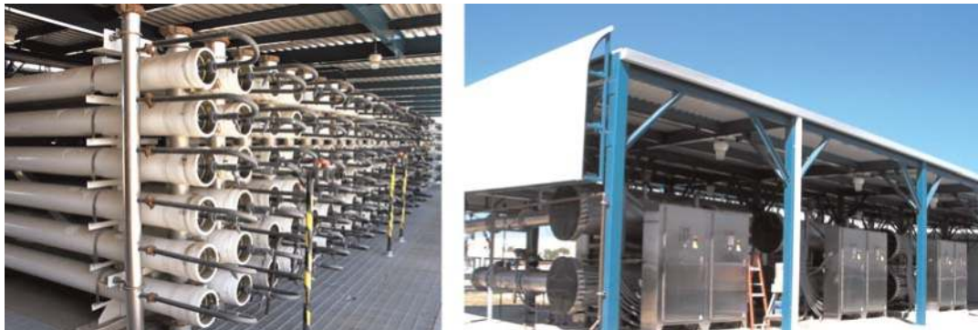
Figure 2.2 View of reverse osmosis and the advanced oxidation by UV/H 2 O 2 .
