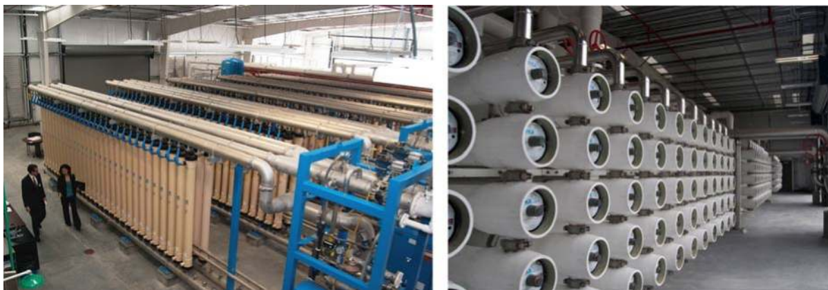
Figure 20.3 Views of the MF system and RO system.
