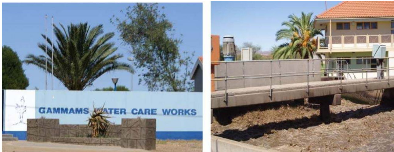
Figure 29.3 View of conventional biological wastewater treatment at the Gammams Water Care Works.
