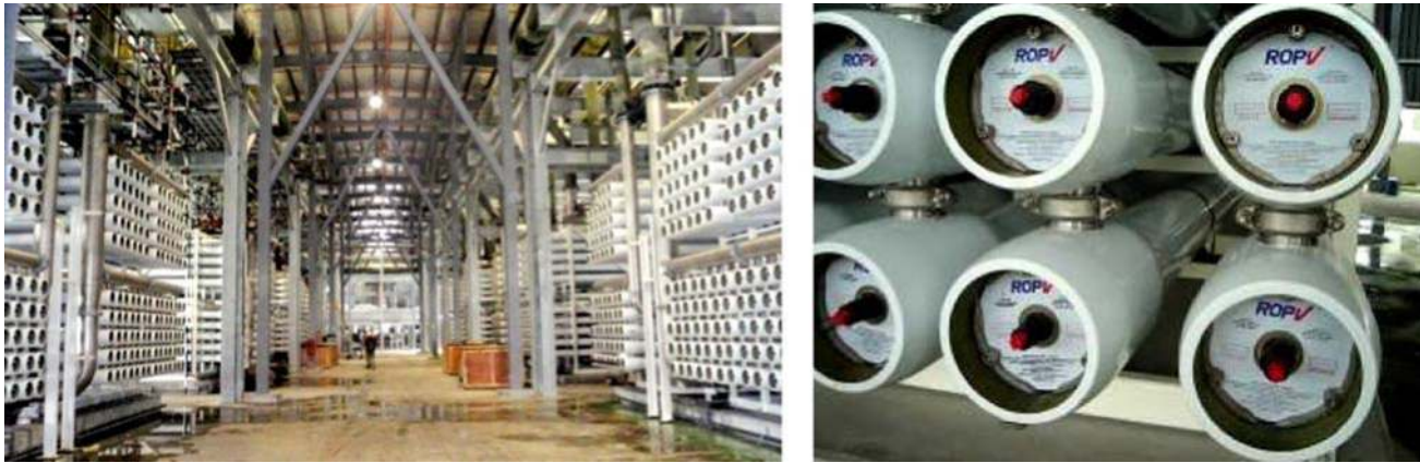
Figure 3.5 NEWater production process: view of reverse osmosis.
