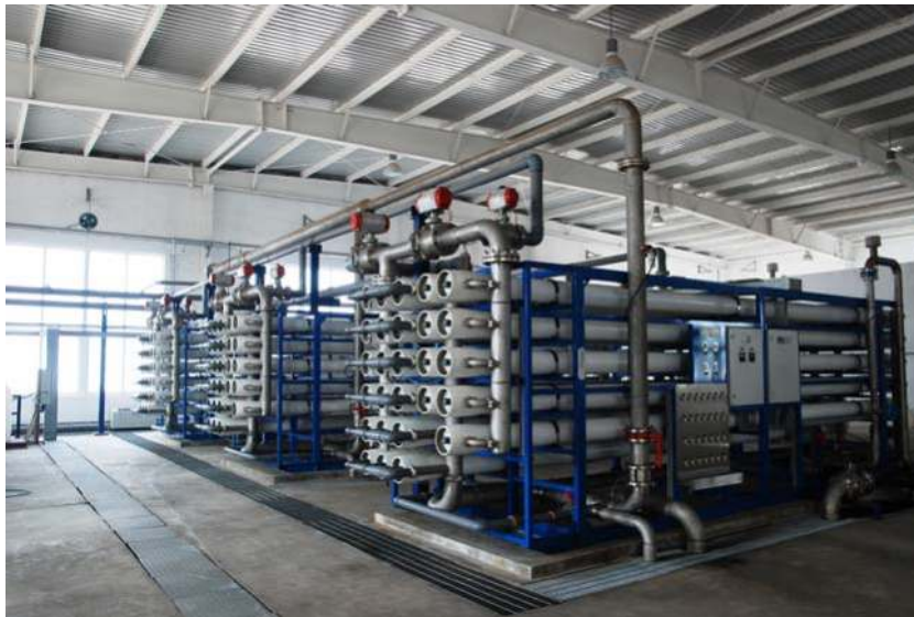
View of the reverse osmosis (RO) technology used to control recycled water salinity in Tianjin.
