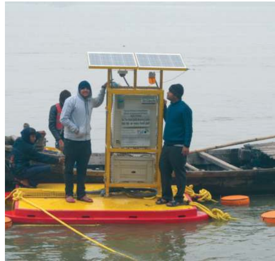
Figure 6.1: Floating monitoring station.
