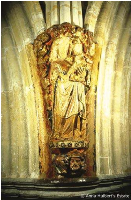
Fig. 1.29 Damaged corbel of Exeter Cathedral. Photograph by Anna Hulbert, no date. Image courtesy of Anna Hulbert's Estate. All rights reserved.
