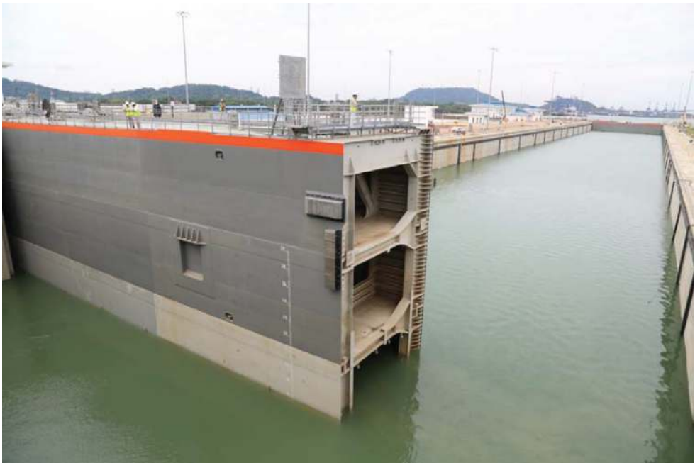
Figure 9. Overview of a gate in operation.
