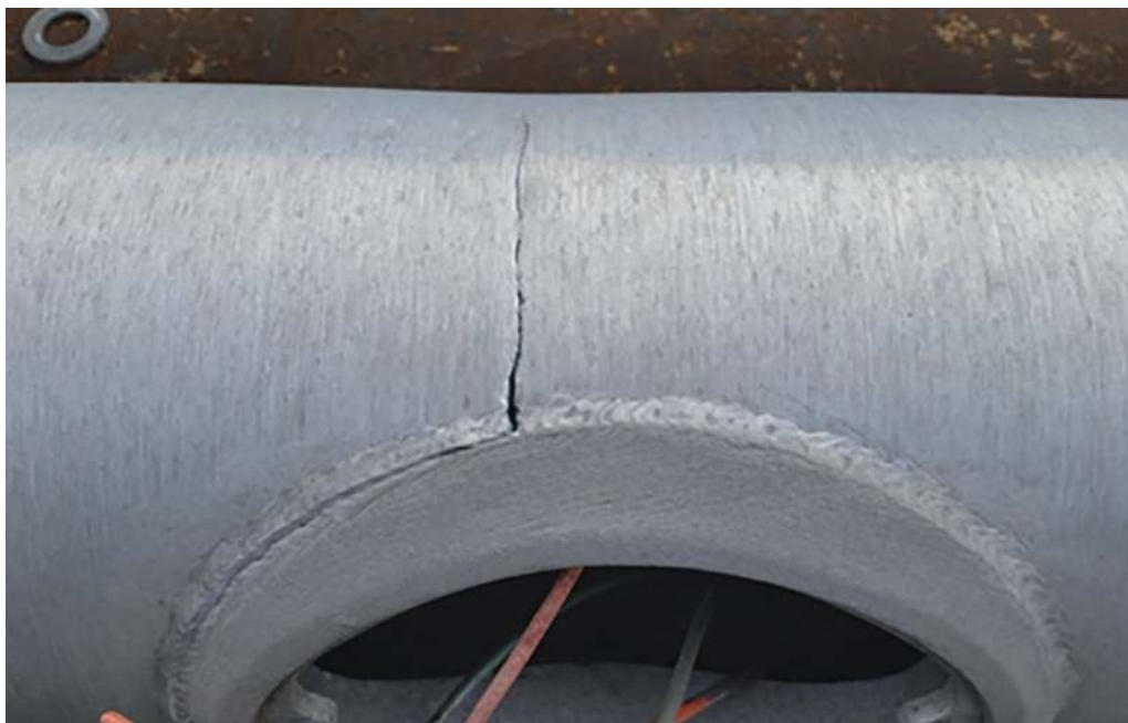
Figure 1. Fatigue crack in welded aluminum light pole hand-hole.
