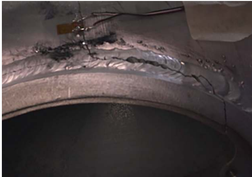
Figure 10. Typical final failure of hand-hole details.
