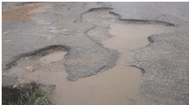
Figure 7. Failed portion in Mission Road.
