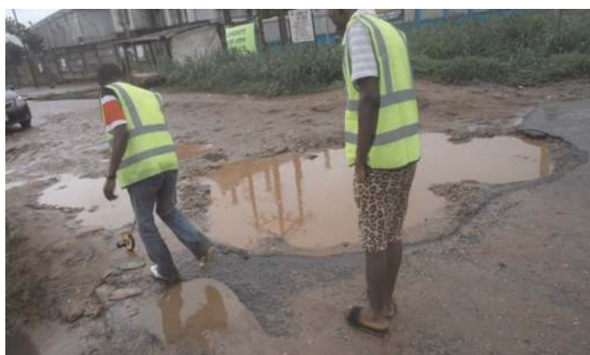
Figure 11. Failed portion in Ogida/Upper Siluko Road.
