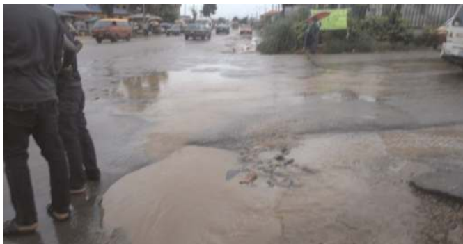
Figure 8. Failed portion in New Benin Road.
