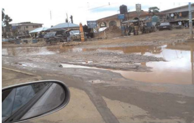
Figure 5. Showing how failed portion of roads affects or increase journey time.
