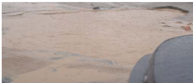
Figure 9. Failed portion in Technical College Road.
