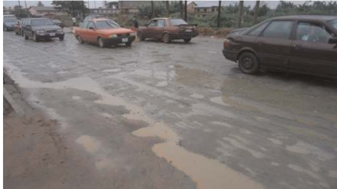
Figure 6. Failed portion in Luckyway Road.
